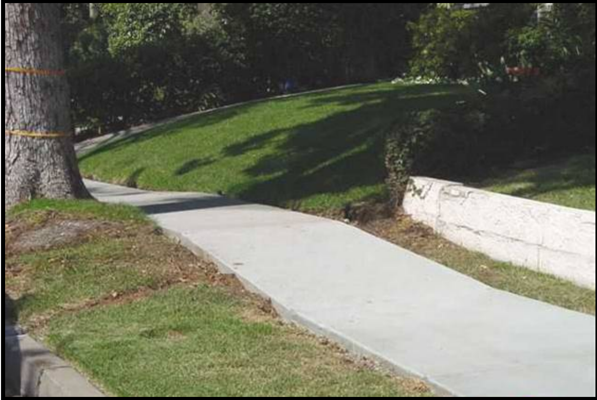
Figure 13 – Sidewalk ramping raises the sidewalk over the root system.
