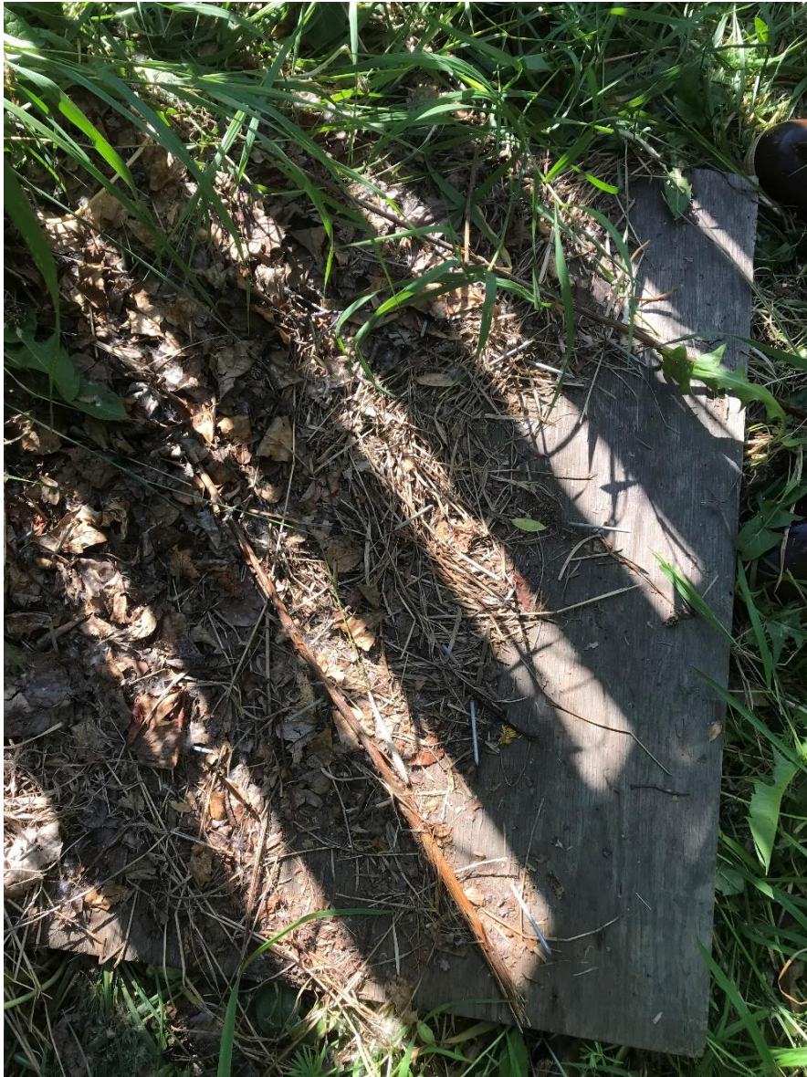
Fish Creek 1277-1. No Safe Access. June 22, 2022.
