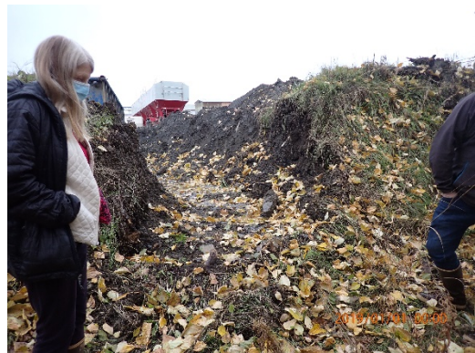
Alaska Stormwater intentional breach in the berm, near creek
