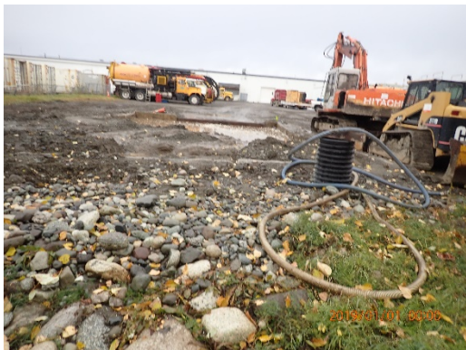
Alaska Stormwater settling tank
