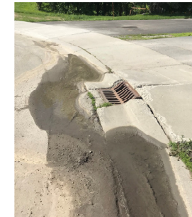
Outfall 555-1 to Fish Creek curbside catch basin frost jacked and not flowing into storm drain
