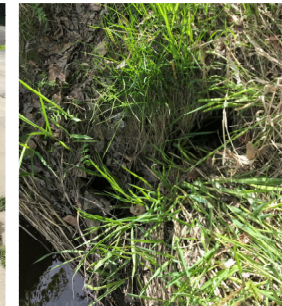
Outfall 703-1 to Campbell Creek is buried by sediment and vegetation
