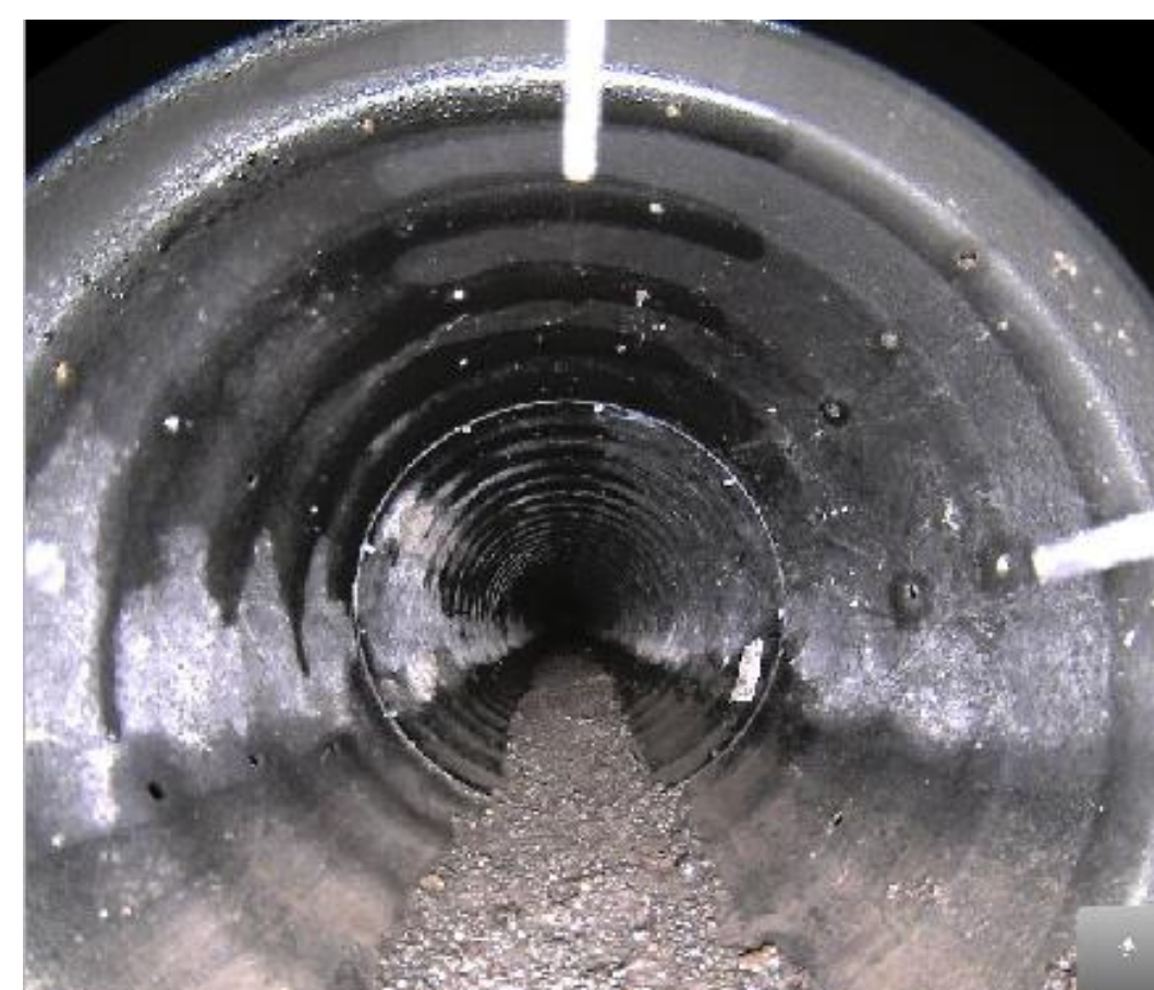
From left to right: Examples of CCTV pictures of pipes in good, moderate, poor, and failing conditions.
