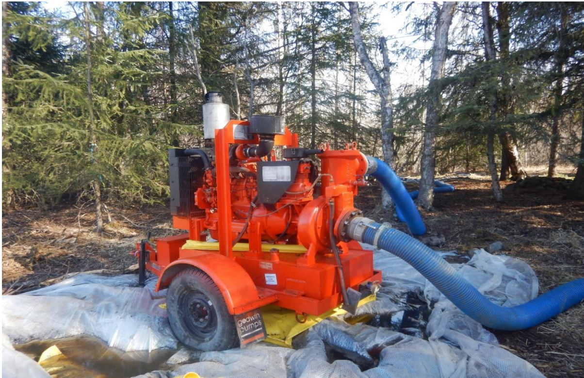
Figure 4. Water pump, Bear Creek.
