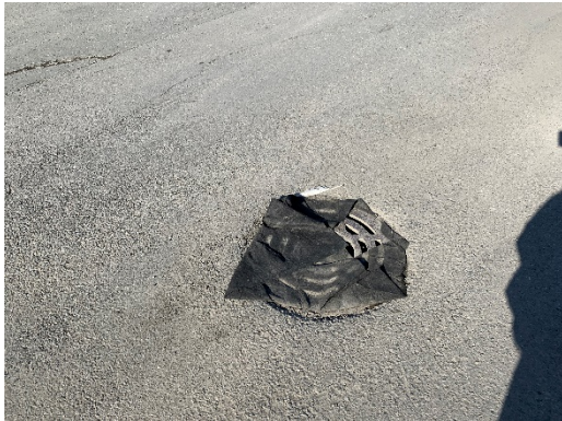
Witches Hat Used in Storm Drain
