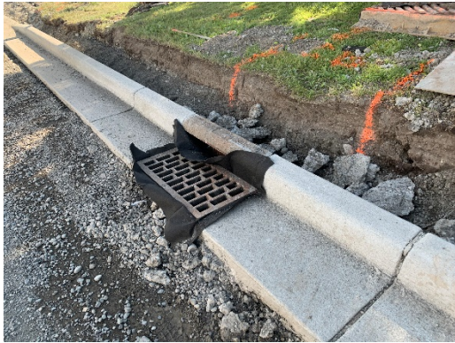
Witches Hat Used in Storm Drain
