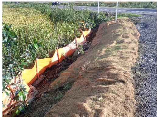
Pullout adjacent to Potters Marsh. The vegetative buffer between the pavement and stone and the marsh has been reestablished, facing north.
