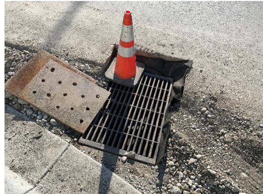
Witches Hat Used in Storm Drain
