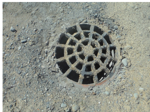
Witches Hats Pulled From Storm Drains As Part Of Winter Shutdown, Will Be Replaces As Construction Resumes
