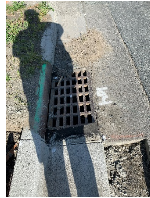
Witches Hat Used in Storm Drain
