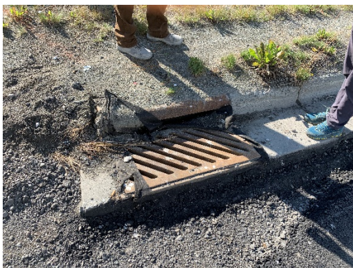
Witches Hat Used in Storm Drain
