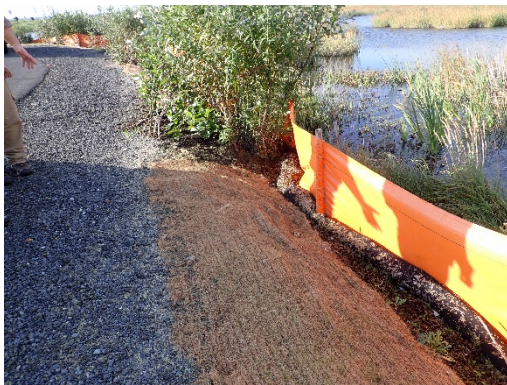
Pullout adjacent to Potters Marsh. BMPs remain in place, facing south. No evidence of sediment or gravel entering the marsh.
