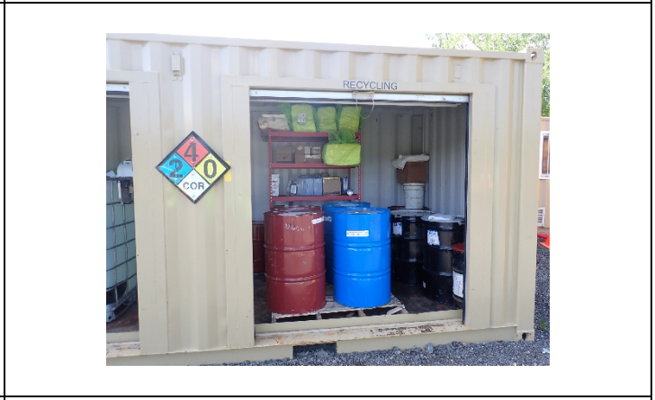
Chemical Storage – 12 of 20
