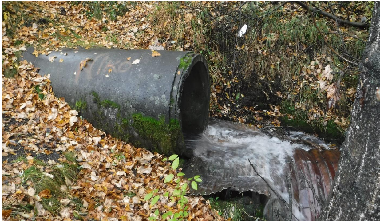
Photograph 8. Outfall SWM08 (86-1), New Seward Highway at Chester Creek.
