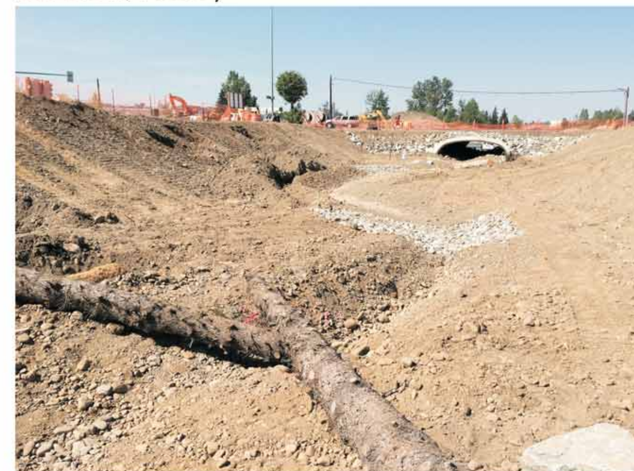
Newly aligned channel just east of Muldoon with meanders and woody debris that were placed to improve stream substrate. (HDR, 2015)
