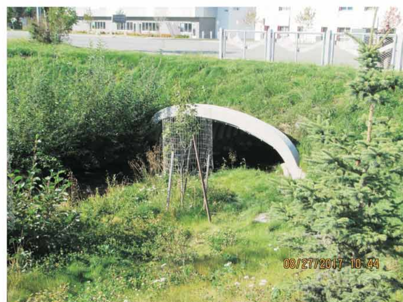
Two years after completion, the vegetation around the culvert (looking west towards Muldoon) is well established. (C. Northon, 2017)
