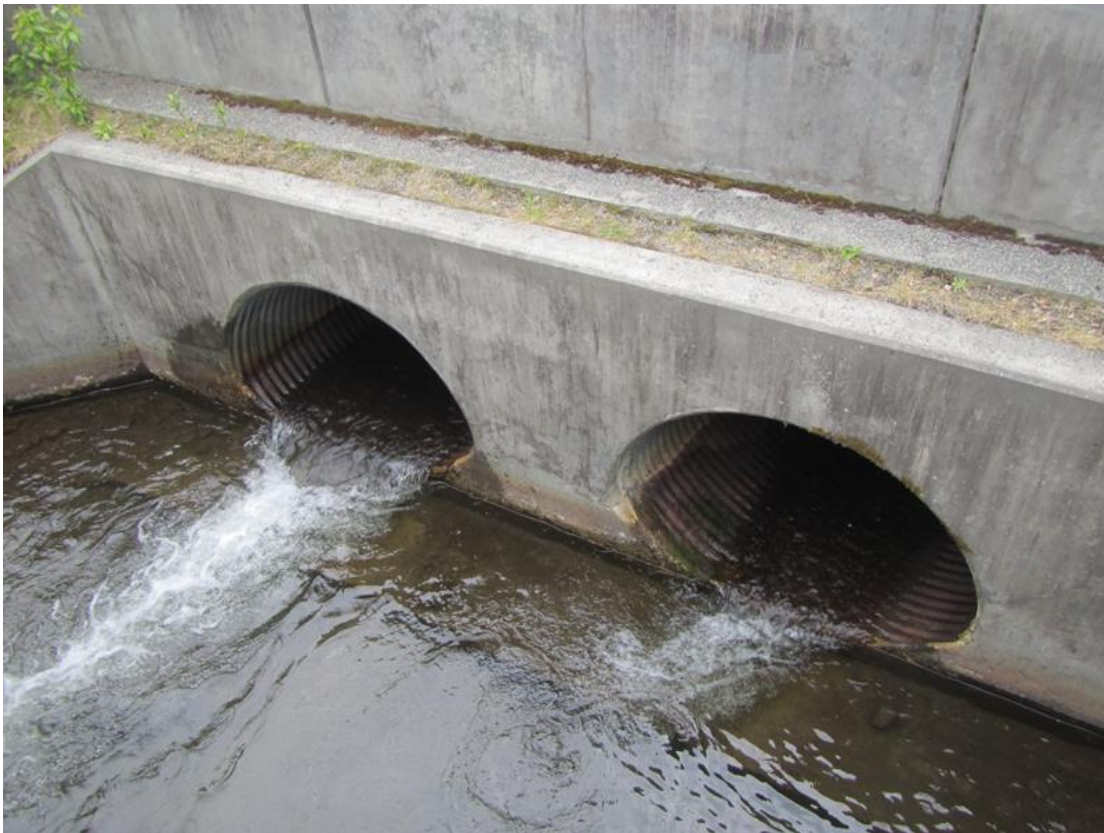
Figure 6 – Outflow culvert (ADF&G #20400085) on the North Fork of Campbell Creek (Photo by T. Eley, 2017)
