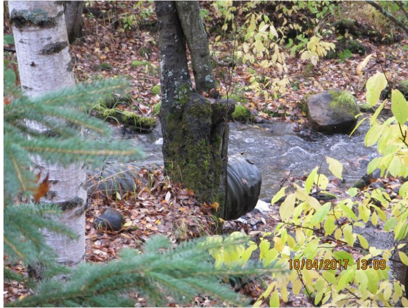
Figure 15. Culvert returning zoo runoff to South Fork of Little Campbell Creek 4 October 2017. (Photo by C. Northon)
