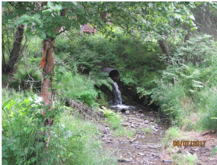
Figure 11. Perched culvert just east of the Alaska Zoo's boundary, South Fork Little Campbell Creek, Anchorage, 2017 (Photo by T. Eley).
