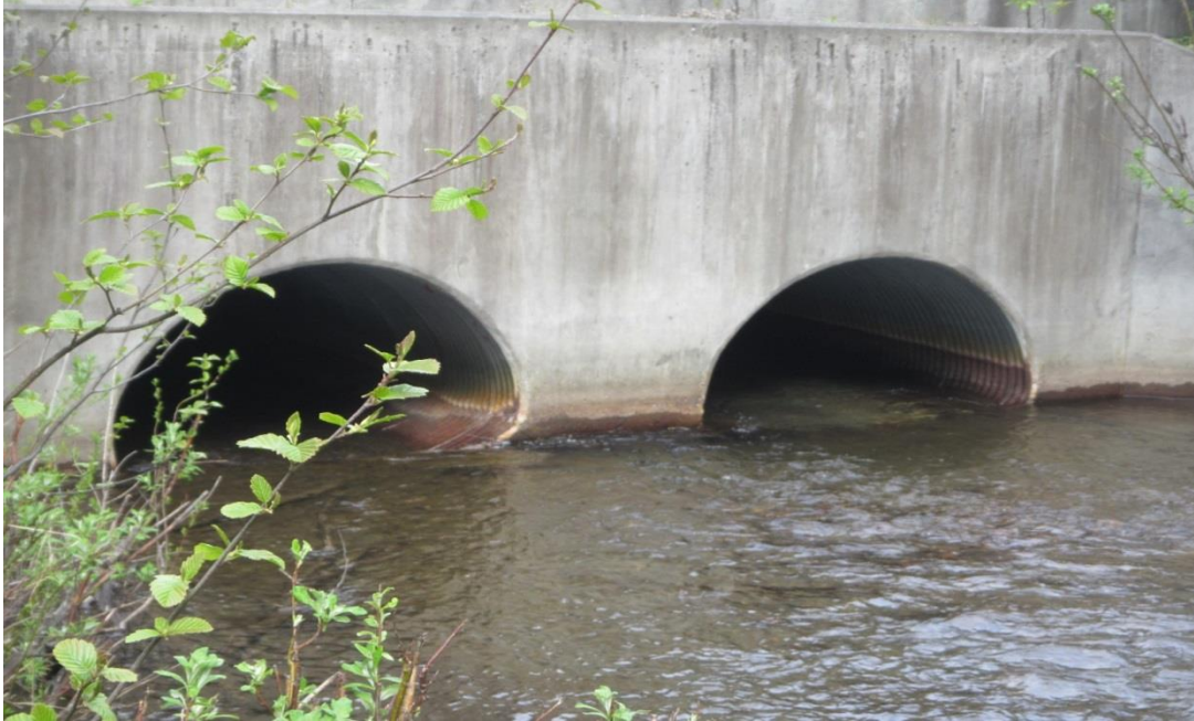
Figure 5 – Inflow culvert (ADF&G #20400085) on the North Fork of Campbell Creek (Photo by T. Eley, 2017)
