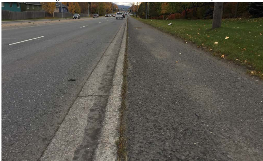
Figure 4.2 – Muldoon Road after the fall sweep.
