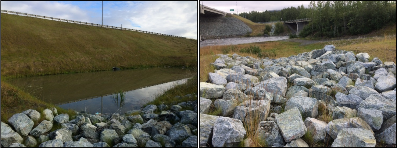
Figure 31: North Detention Pond (left) and Spillway Outfall from South Detention Pond (right), August 8, 2018
