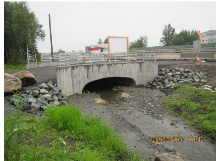
View of the new driveway over N. Fork Little Campbell Creek looking north (2017).
