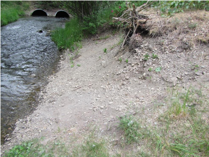
Bank erosion in 2013 on north side of Chester Creek near Elmore
