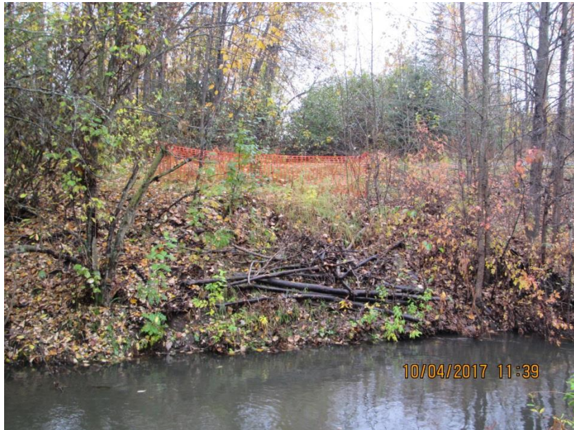
2014 bank restoration shown in 2017 on south side of Chester Creek near Elmore
