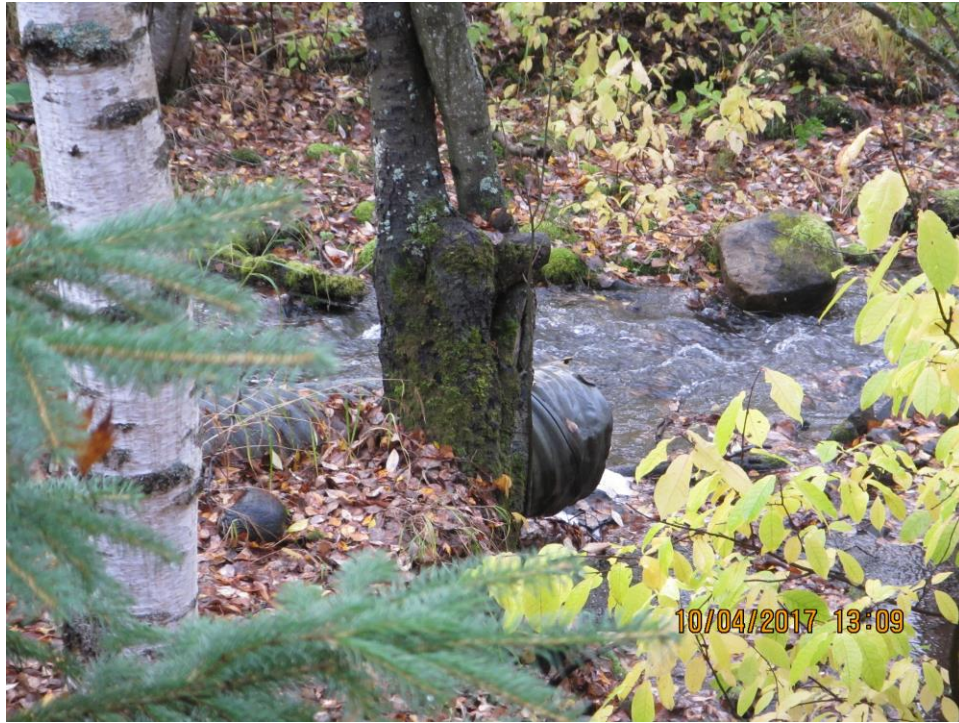
Photo 5. Culvert returning water from the brown bear exhibit to Little Campbell Creek. (Photo by Cherie Northon)
