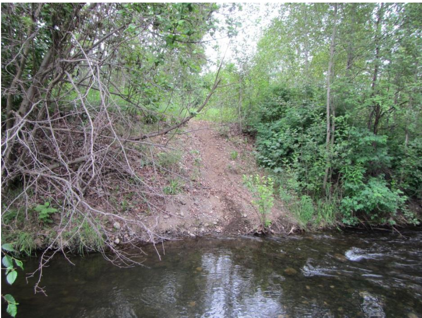
Bank erosion in 2013 on south side of Chester Creek near Elmore
