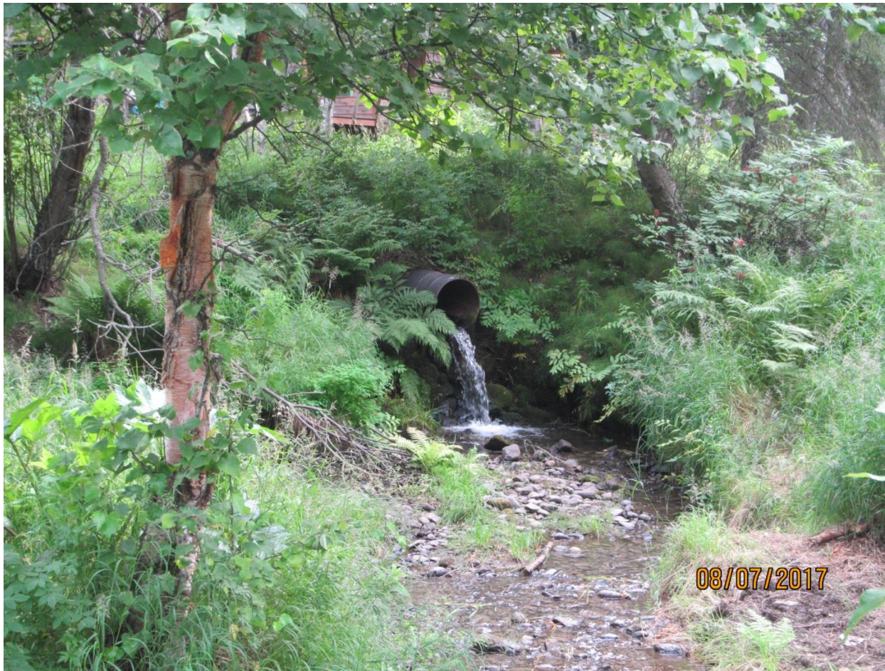
Photo 1. Perched culvert just east of the Alaska Zoo’s boundary, Little Campbell Creek, Anchorage (2017) (Photo by Thom Eley).
