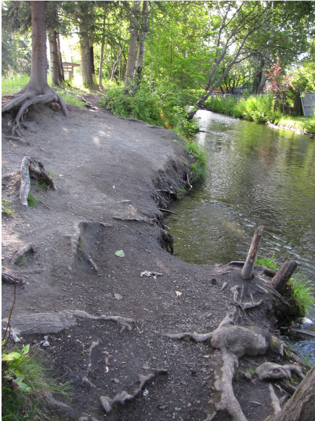
West bank of Chester Creek showing eroded bank in 2011 (CW-4)
