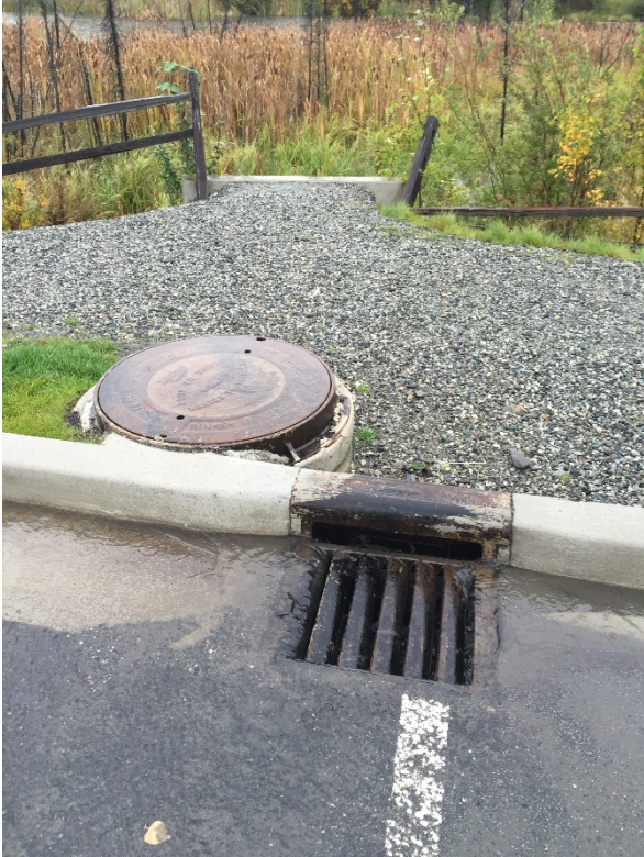
Catch basin on south side of pond (from Cabelas lot).
