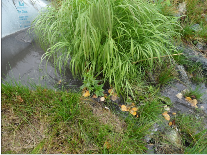
Inflow partially blocked by vegetation.
