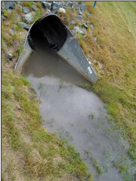
Bioswale outfall – flowing slowly.
