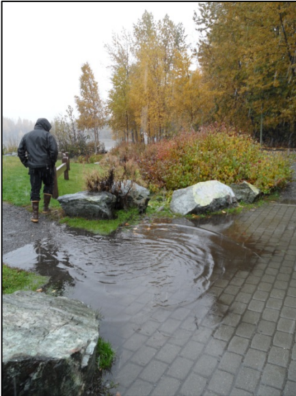
Ponding at the rain garden inlet
