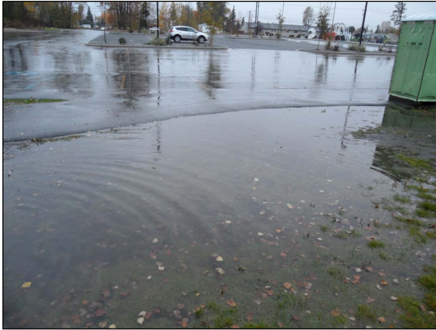
Figure 23: Ponding on the East Side of Parking Lot
