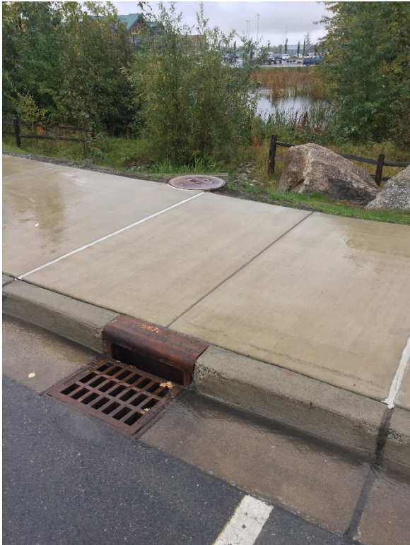
Catch basin on north side of pond, leading to culvert and discharge into pond.
