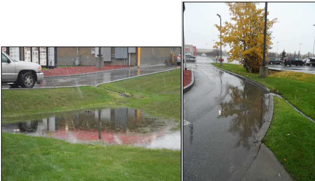
Left: overflow beehive that is not flowing. Right: Ponding and outflow of McDonald's Drive through
