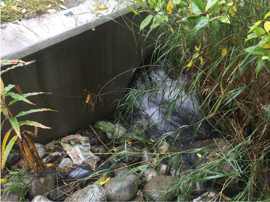
Flow from culvert connected to catch basin at north side of pond (Target parking lot).
