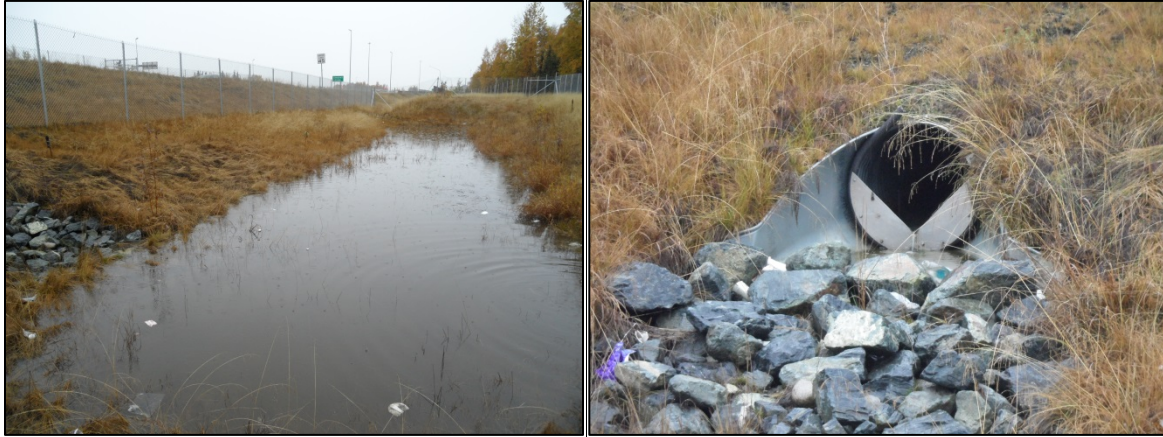
Left: Ponding in the facility. Right: Inlet actively flowing.
