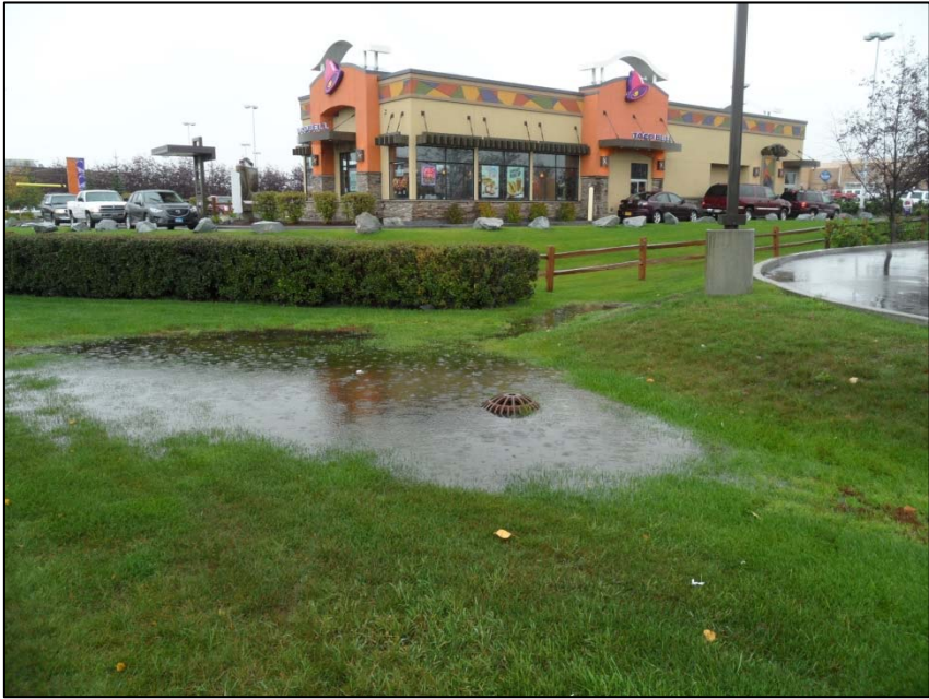
Figure 36: Ponding in Swale Low Point
