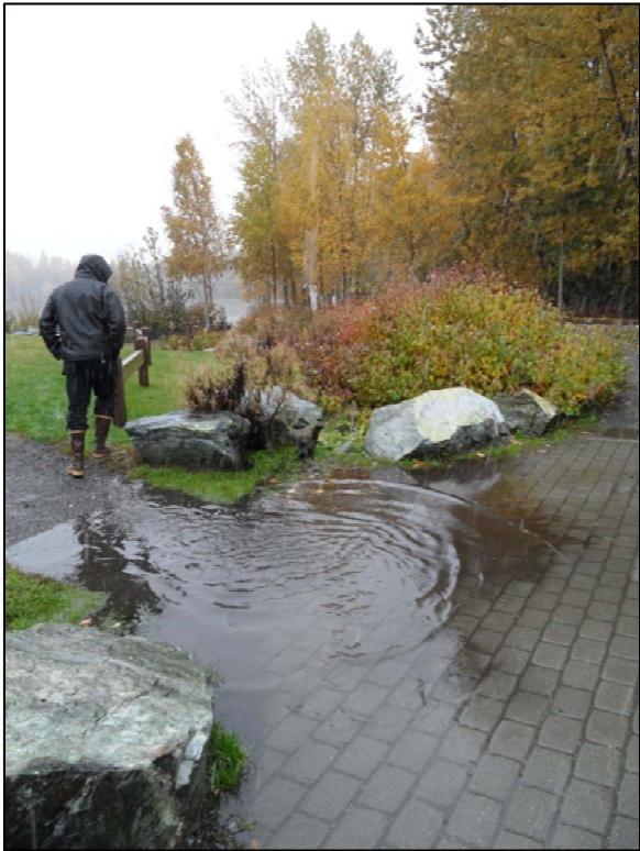
Figure 27: Ponding Near the Inlet 9/29/15
