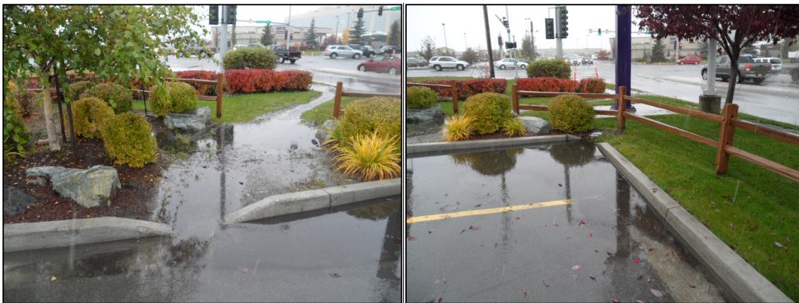
Taco Bell Parking Lot – North Side. Foot path overflowing.
