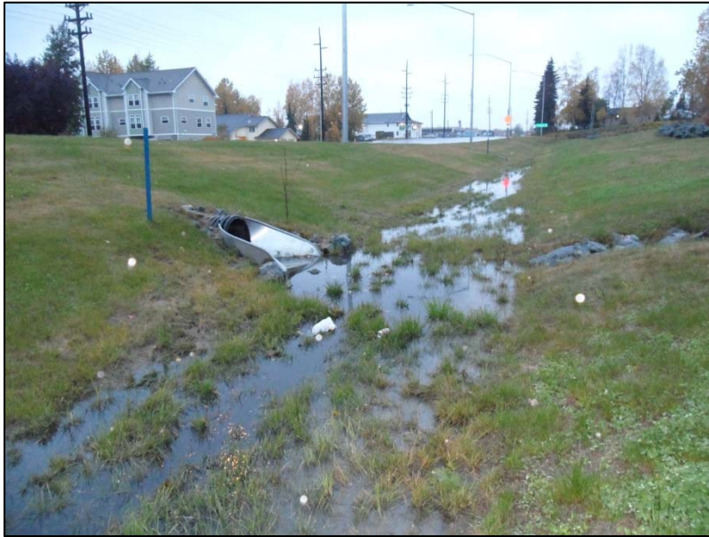
Figure 6: Bioswale Overview on 9/29/15
