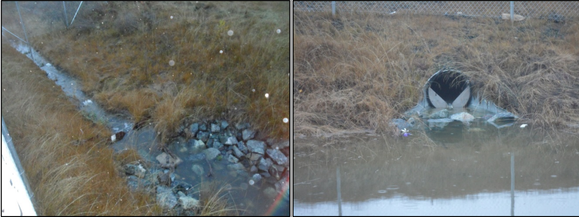
Left: Facility outlet. Right: Facility inlet
