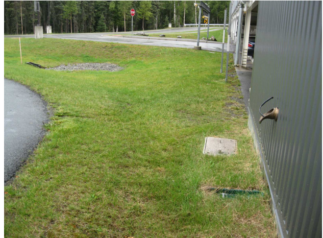
2 scupper on west side of ANSEP bldg. between Areas #2 and #3 on site plan
