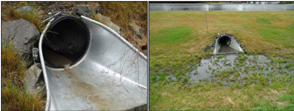
Inflow to bioswale and ponding at storm drain inflow pipe.
