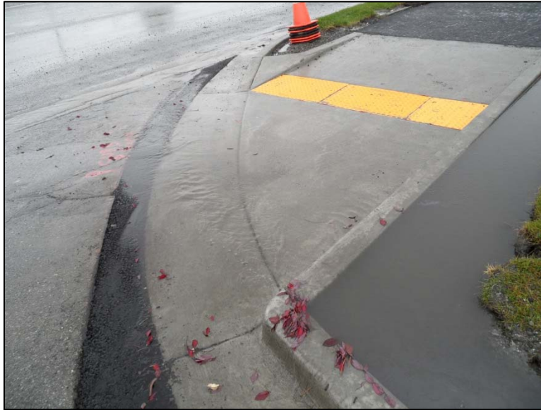
Figure 32: Overflow Along North Side of Holiday Rain Garden
