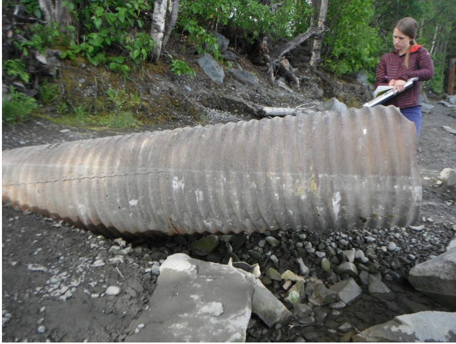
Ship Creek 119-1 : Jacked up and rusted out.
