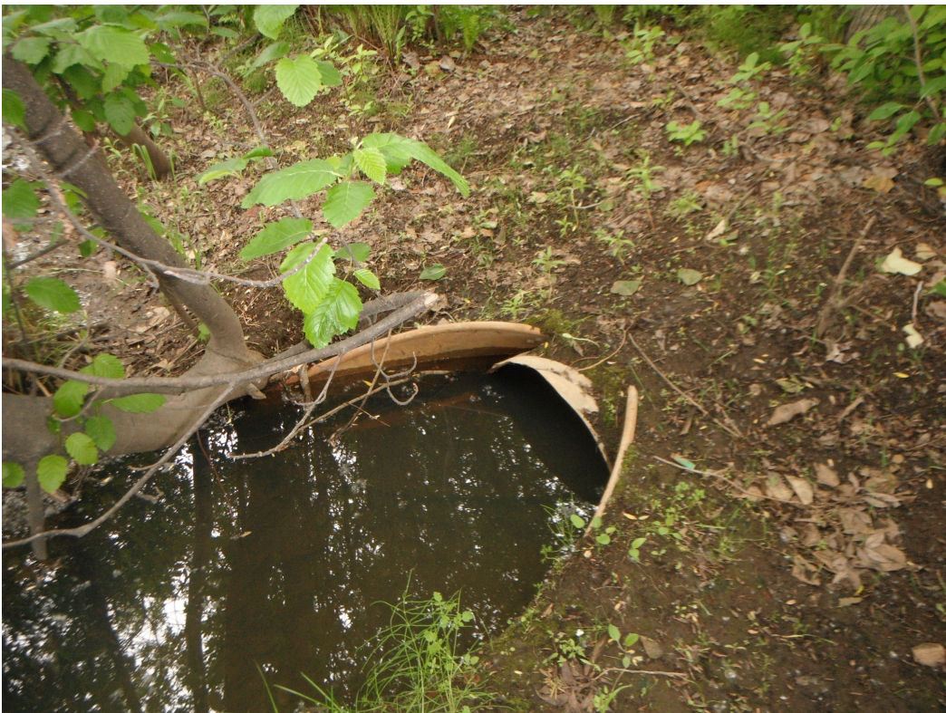
Fish Creek 391-1 : End of pipe damaged and submerged
