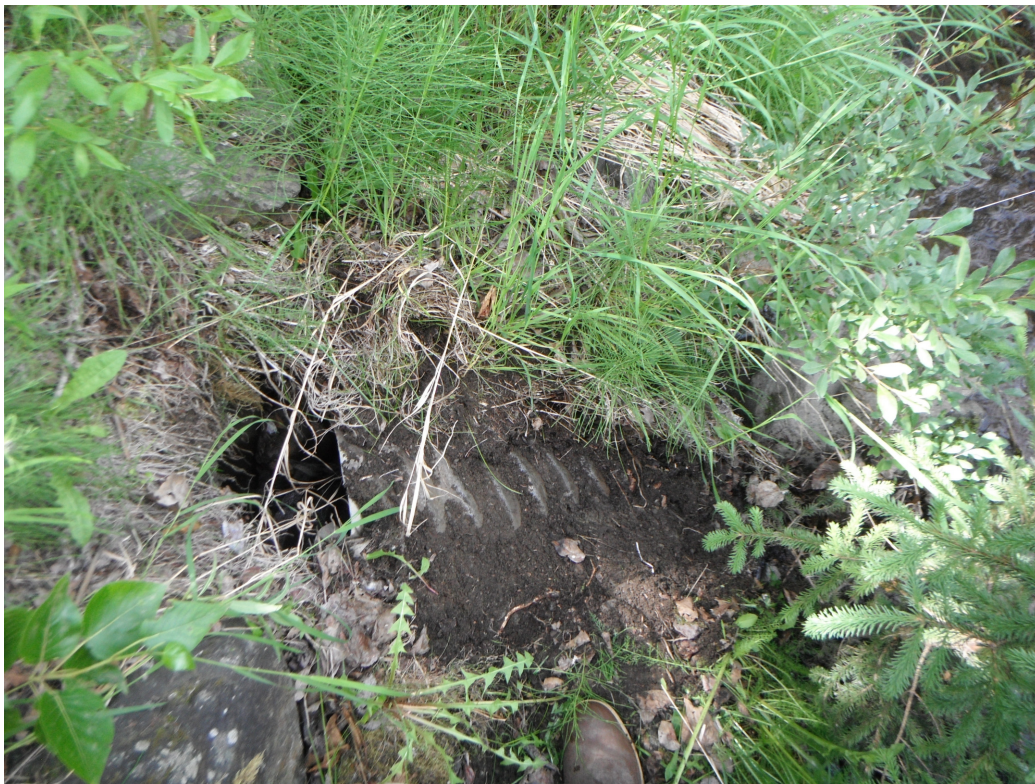
Campbell Creek 447-64 : Broken and bent. Note Creek to right, outfall flowing, but is inaccessible
