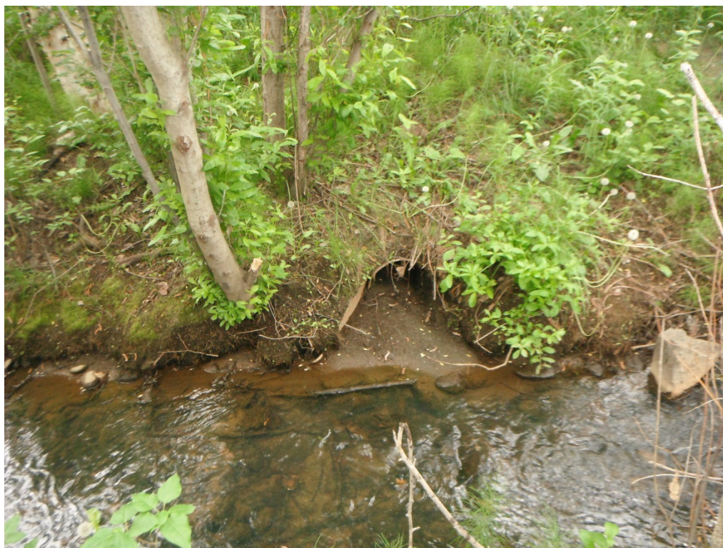
Fish Creek 1277-59 : Clogged with sediment
