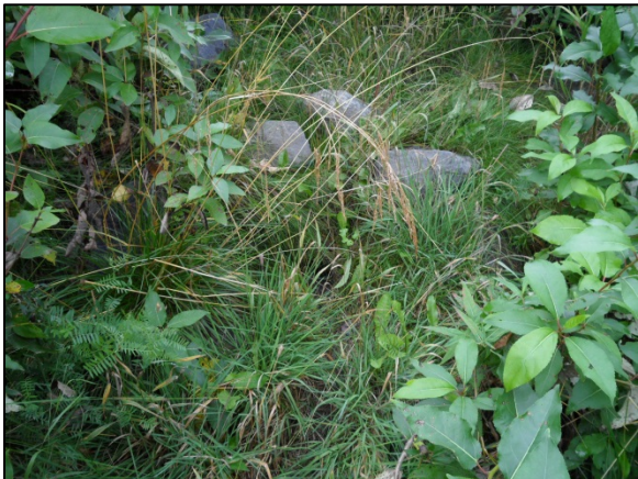
Outlet pipe with no flow
