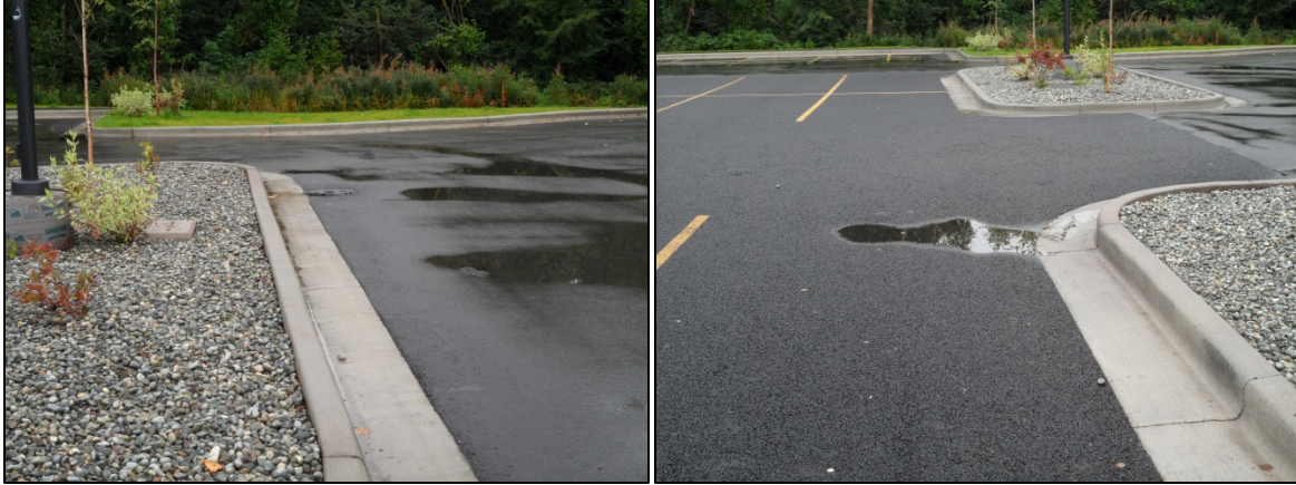
Left: New rock mulch. Right: ponding on the porous asphalt surface
