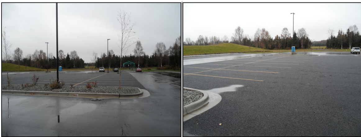
Left: Parking lot overview. Right: ponding on the porous asphalt
