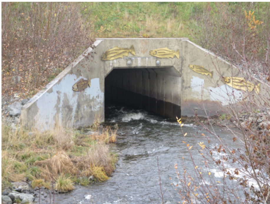
New box culvert passage between Westchester and Cook Inlet, which allows a direct connection thus restoring tidal flushing and wetland habitat to nearly 5 acres of the original 60-acre estuary (photo by C. Northon)
