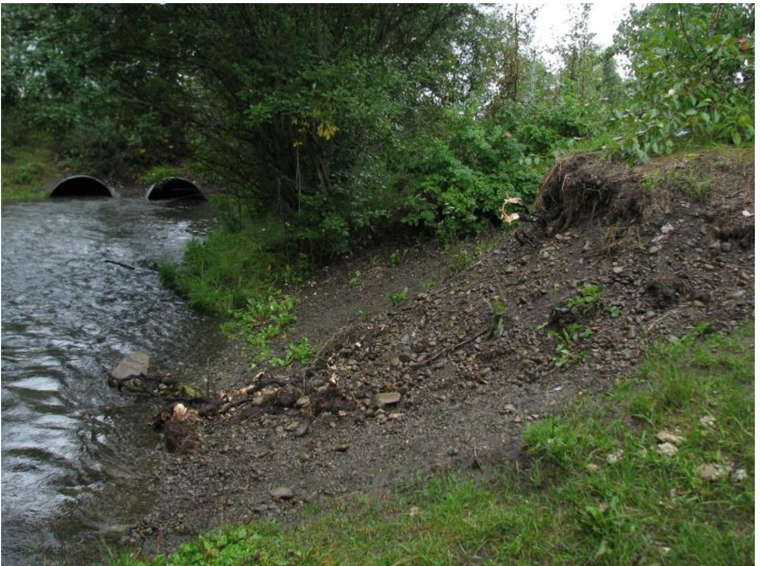
Bank erosion most likely from human foot and bike traffic on the South Fork of Chester Creek by Elmore (M. Houser)
