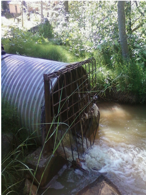
Fish Creek (1288-1) Large culvert in Hermit Park. End of piped branch of creek which is used as a storm sewer.
