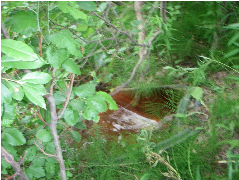
Campbell Creek 120-22-1 South side of Ridgemont Drive near Spruce View Loop. Node code assigned based on location, but not currently in HGDB. Lab report labels this as 344-18-1. Code was updated to 120-22-1 during report mapping.
