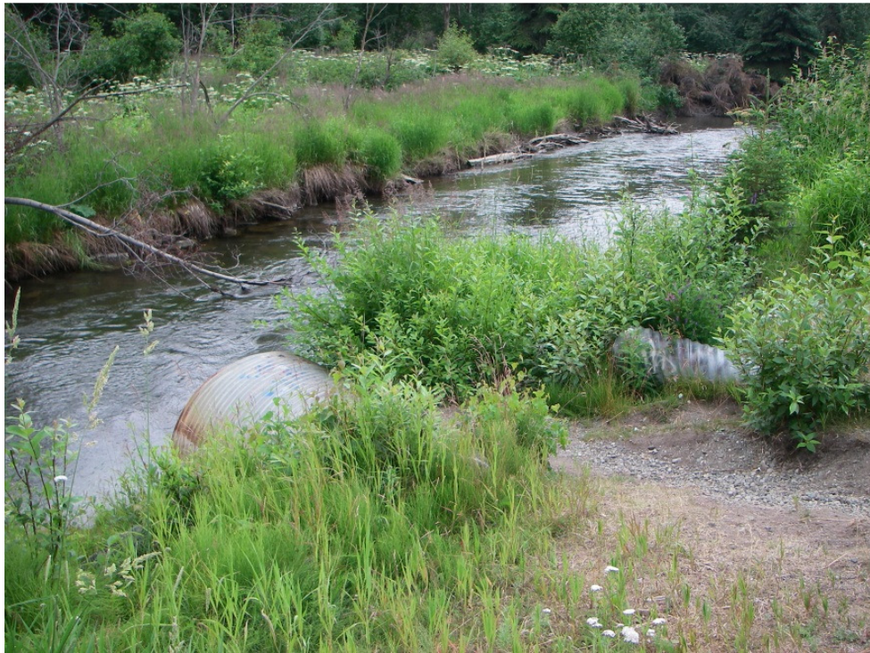
Campbell Creek 651-1 Drains Greenhill Way into creek
