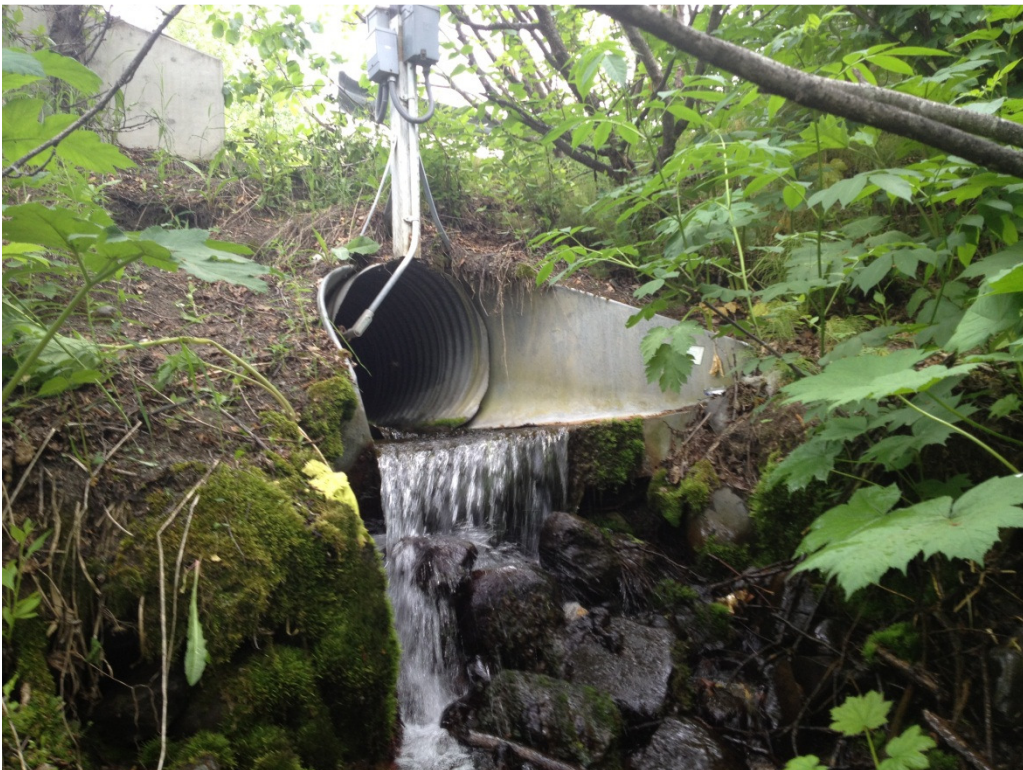
Potter Creek (101-1) South of Potter Valley Rd, east of bridge over creek
