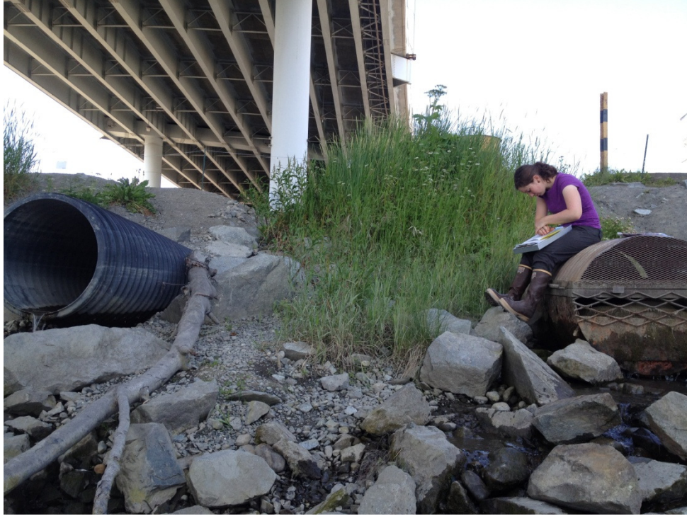
SHP 396-1 (right) Outfall
