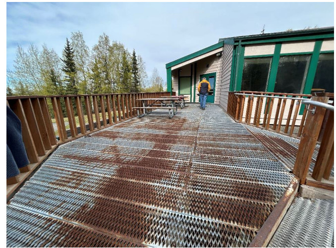
Above: Existing condition of the deck with deteriorating surface.
