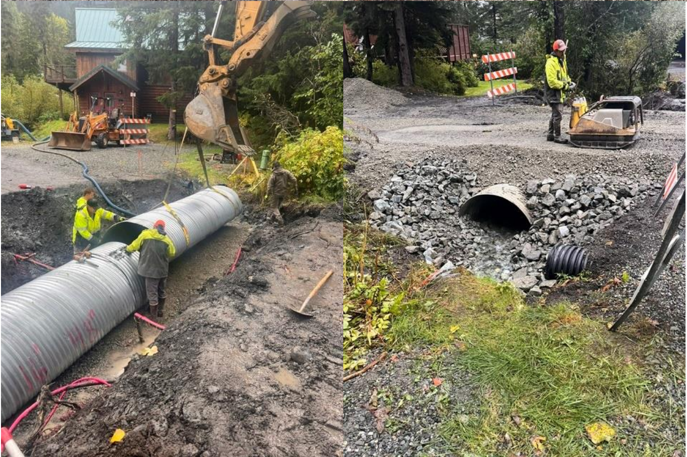
Installing new culvert around all the utilities and working on final product
