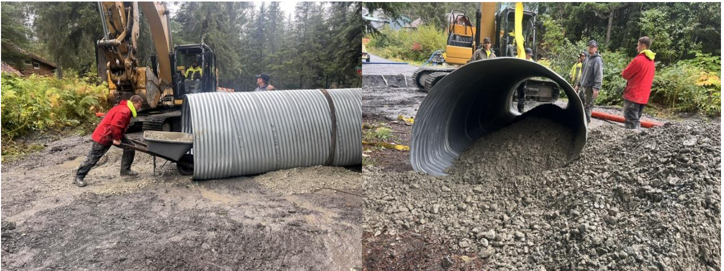
Preloading the culvert with gravel to create a natural bottom for fish to pass over
