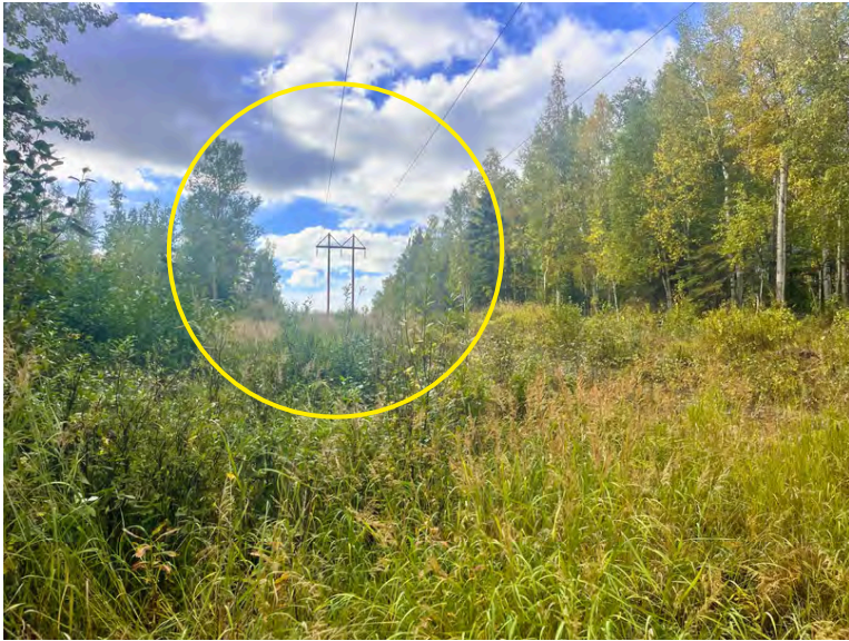
Electrical Transmission Lines, West View
