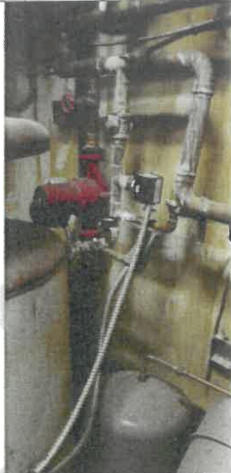
13.0-2: Existing Boiler Room Piping
