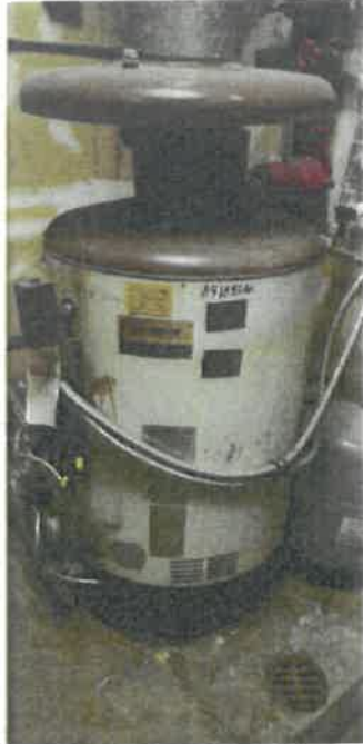
13.0-1: Existing Residential Wing Boiler
