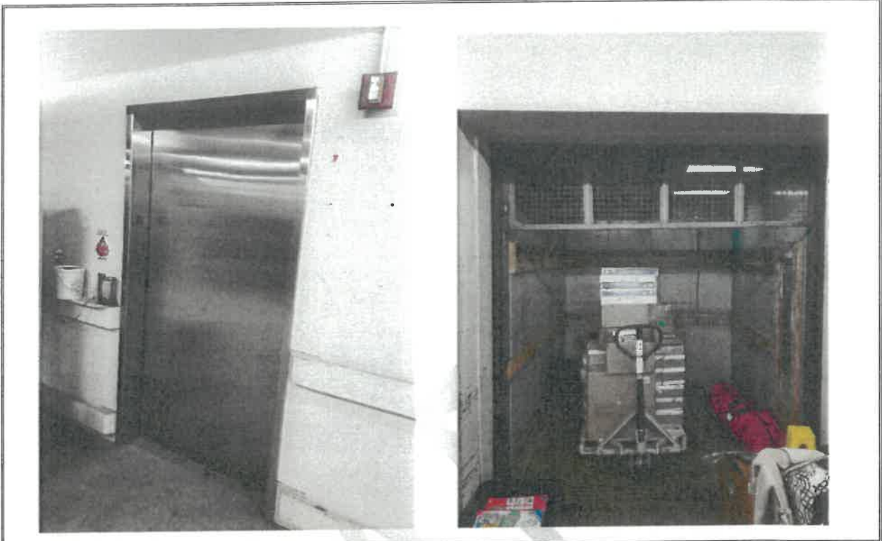
Photos 15.0-1 & 2: Passenger Elevator and Freight Elevator.
