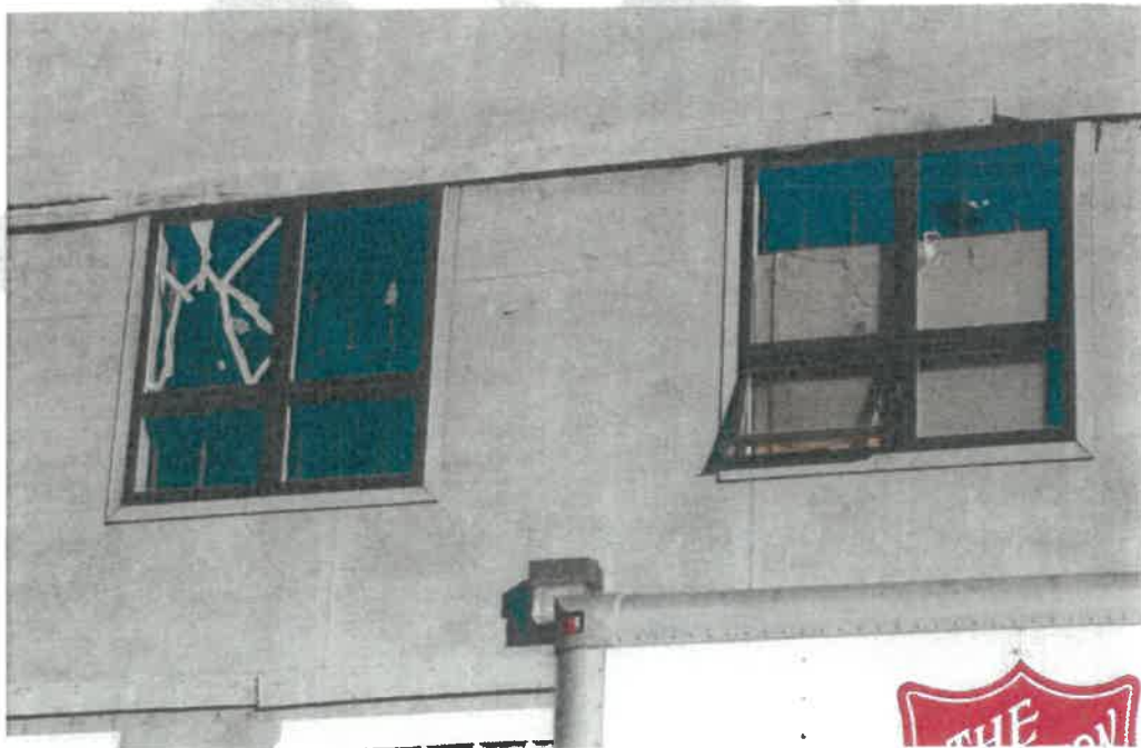
Photograph 10.2-1 – Windows with broken glass in the warehouse
