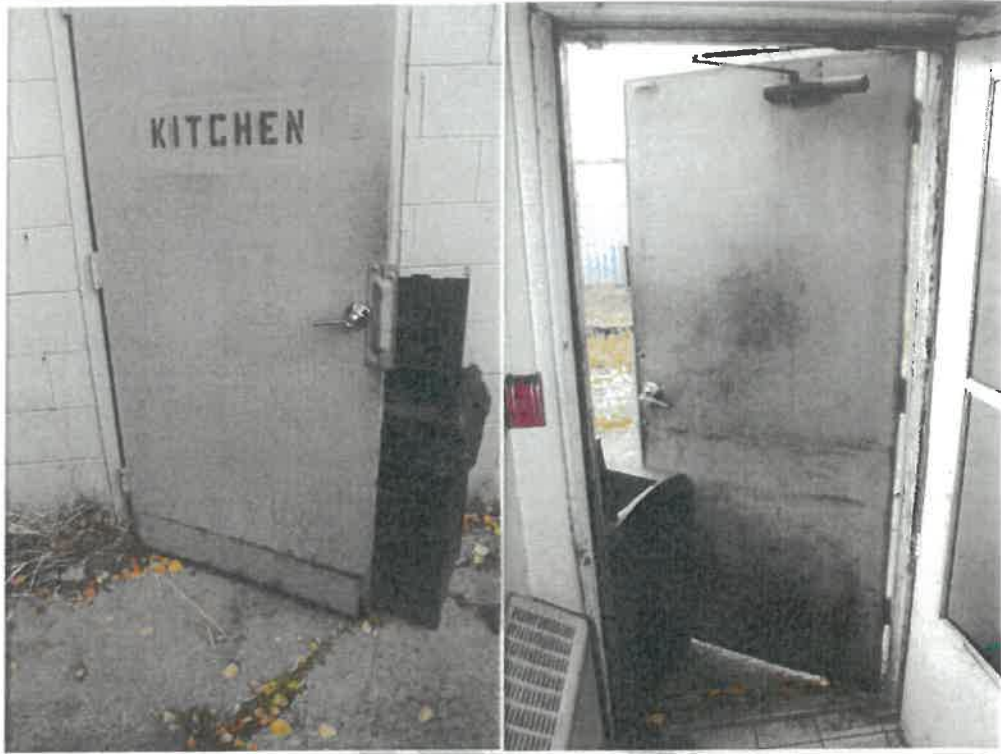
Photograph 10.3-2 – Kitchen door and frame are rusted through
