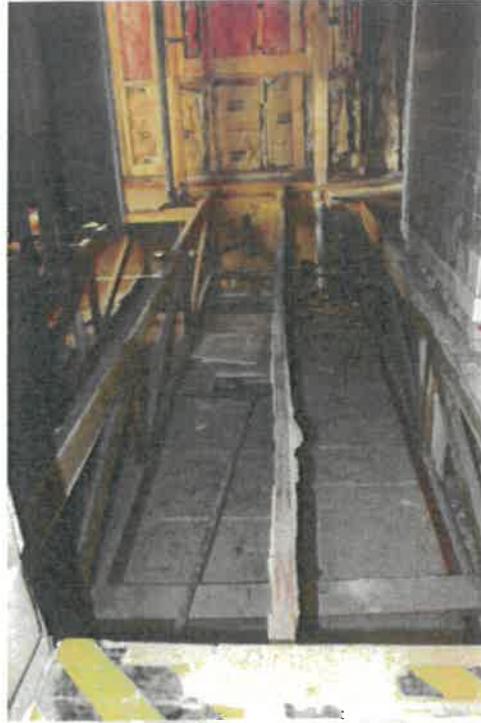
Photograph 9.0-1: Structural Damage, Residential Wing 2 nd Floor
