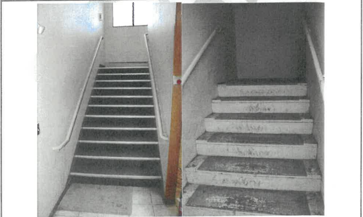
Photograph 17.4-1 – Carpeted main stair (left) and wooden stair in south-west stair enclosure (right)
