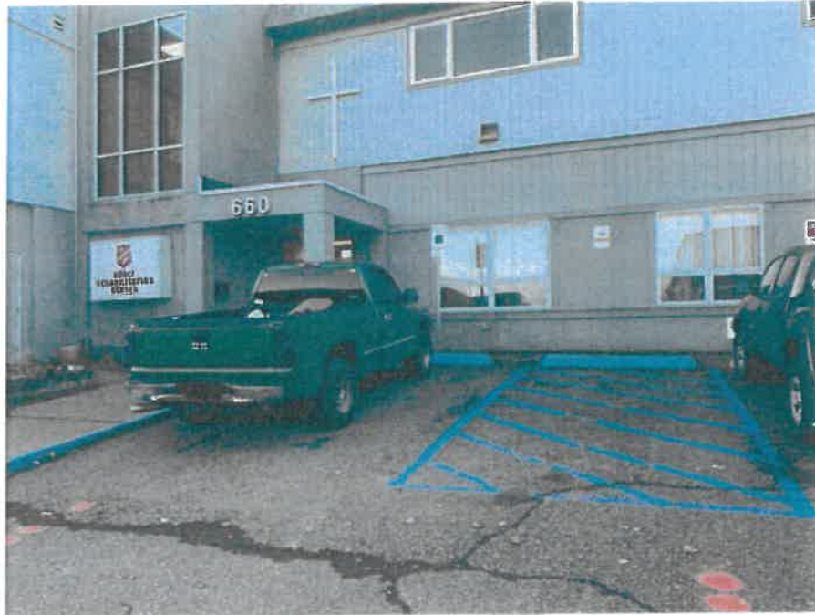
Photograph 6.0-1: Non-compliant ADA parking spaces
