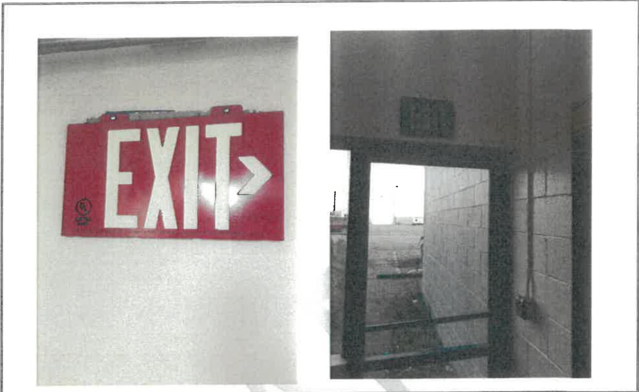
Photos 16.0-10 & 11: Improper Photoluminescent Exit and Expired Nuclear Exit Sign.
