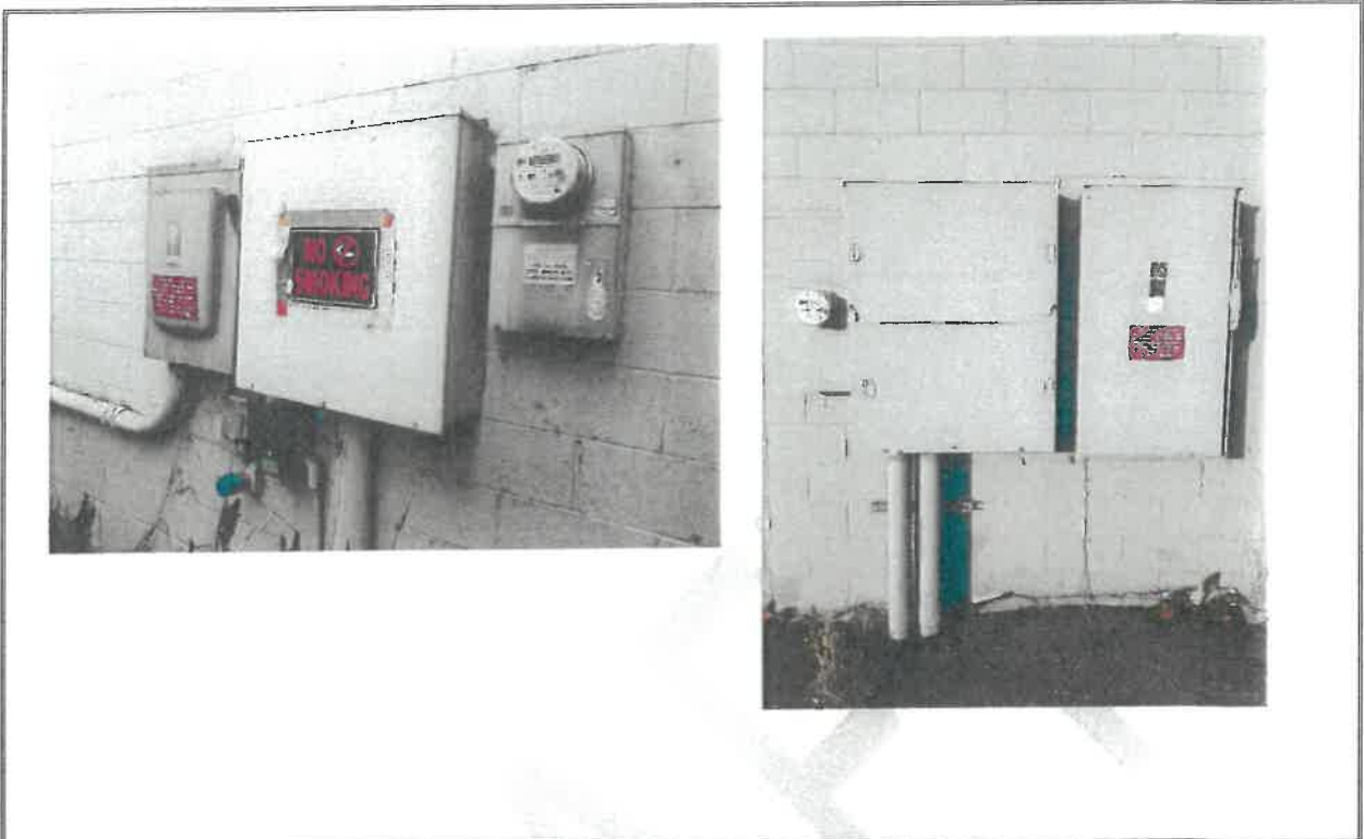
Photos 14.0-1 & 2: 208V and 480V Electrical Service Equipment
