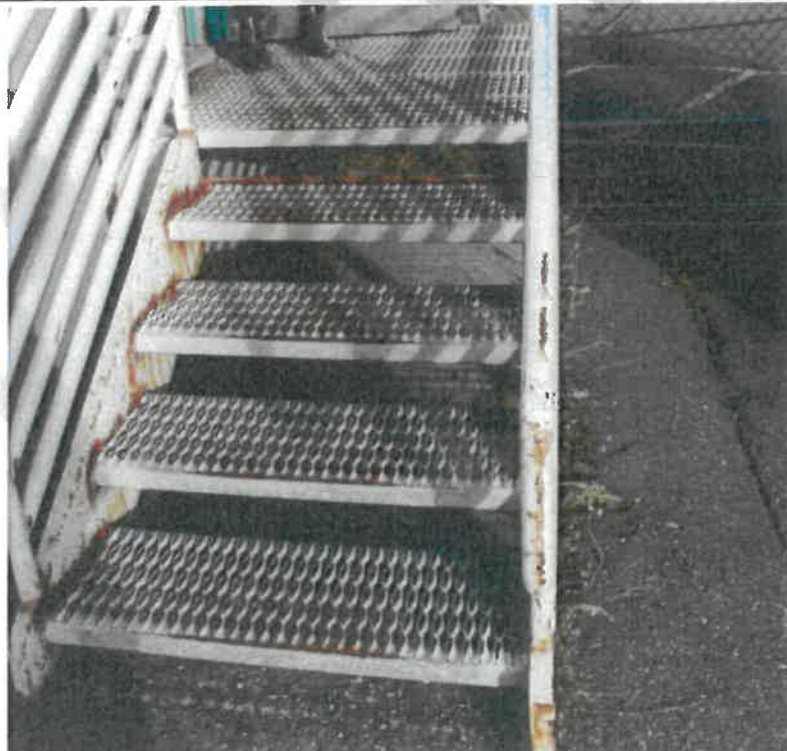
Photograph 10.4-1 – Exterior stair is rusted but serviceable, recommend repainting
