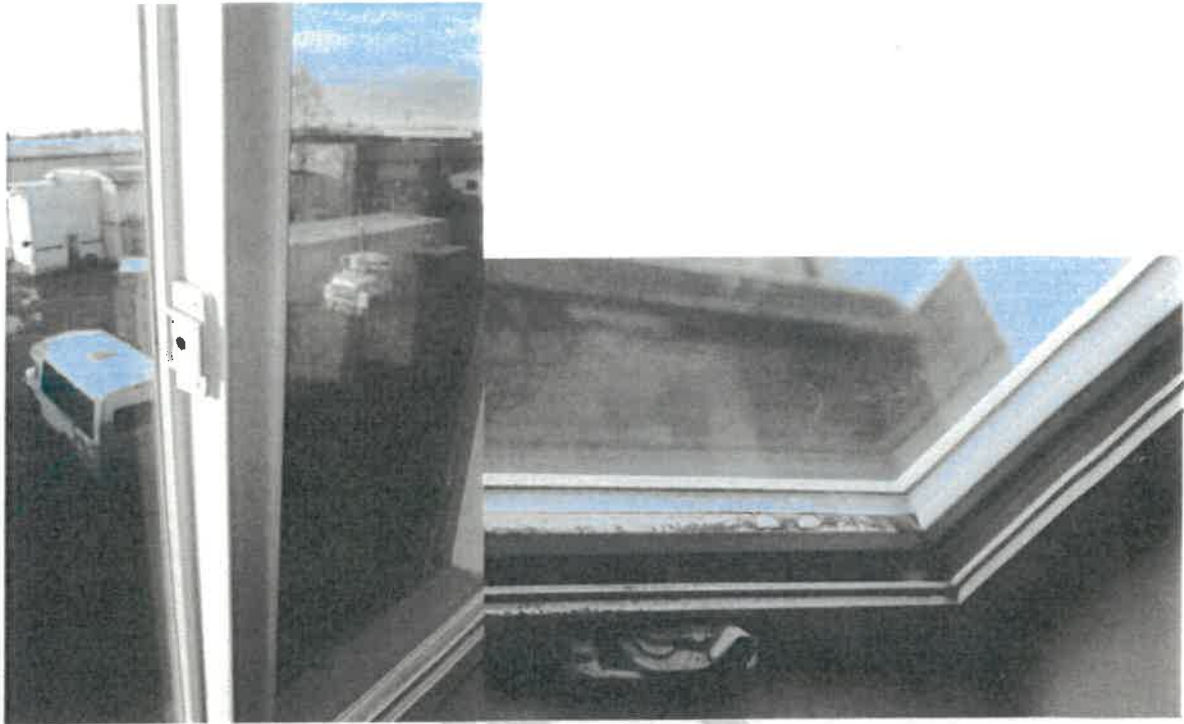
Photograph 10.2-2 – Vinyl windows missing operators (left), Day room window warped (right)
