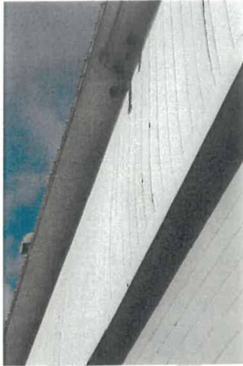
Photograph 10.1-4 – T1-11 wood siding is stained and bowed next to drain pipes
