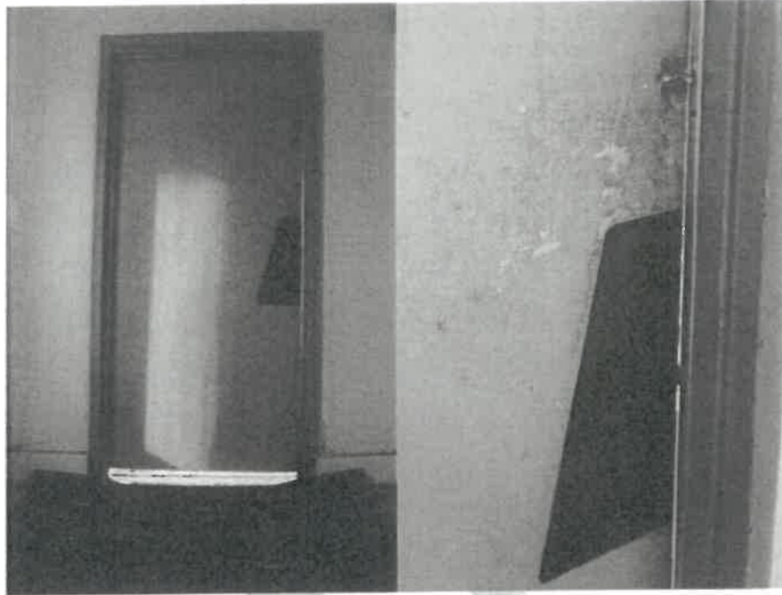
Photograph 5.2-2 – Dining room's south vestibule exit door is undercut and dead-bolted
