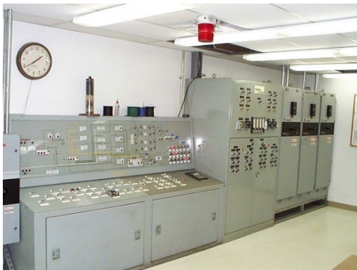
Girdwood Wastewater Treatment Plant
