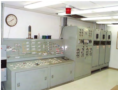
Girdwood Wastewater Treatment Plant
