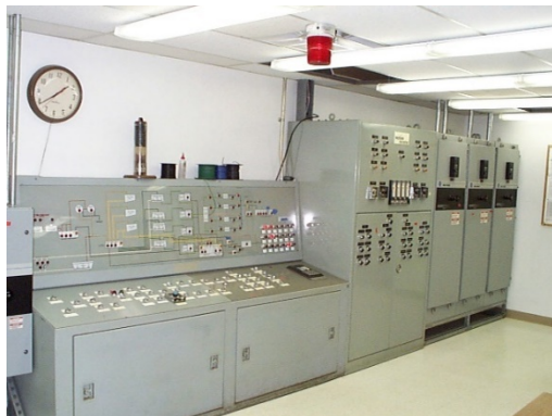
Girdwood Wastewater Treatment Plant
