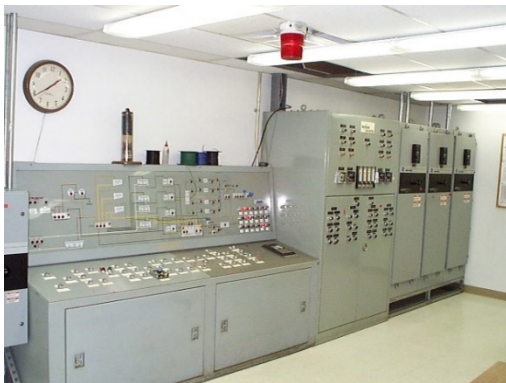
Girdwood Wastewater Treatment Plant
