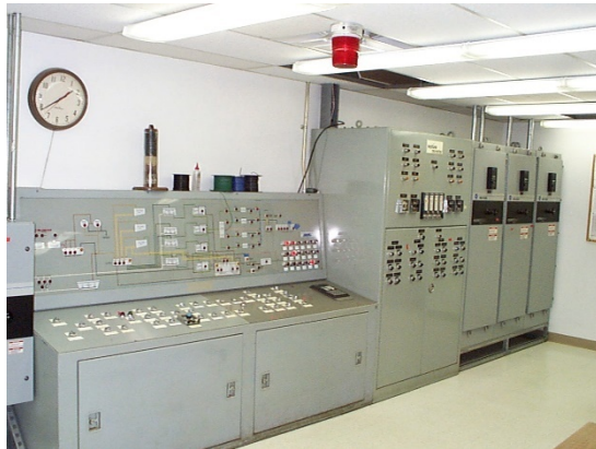
Girdwood Wastewater Treatment Plant
