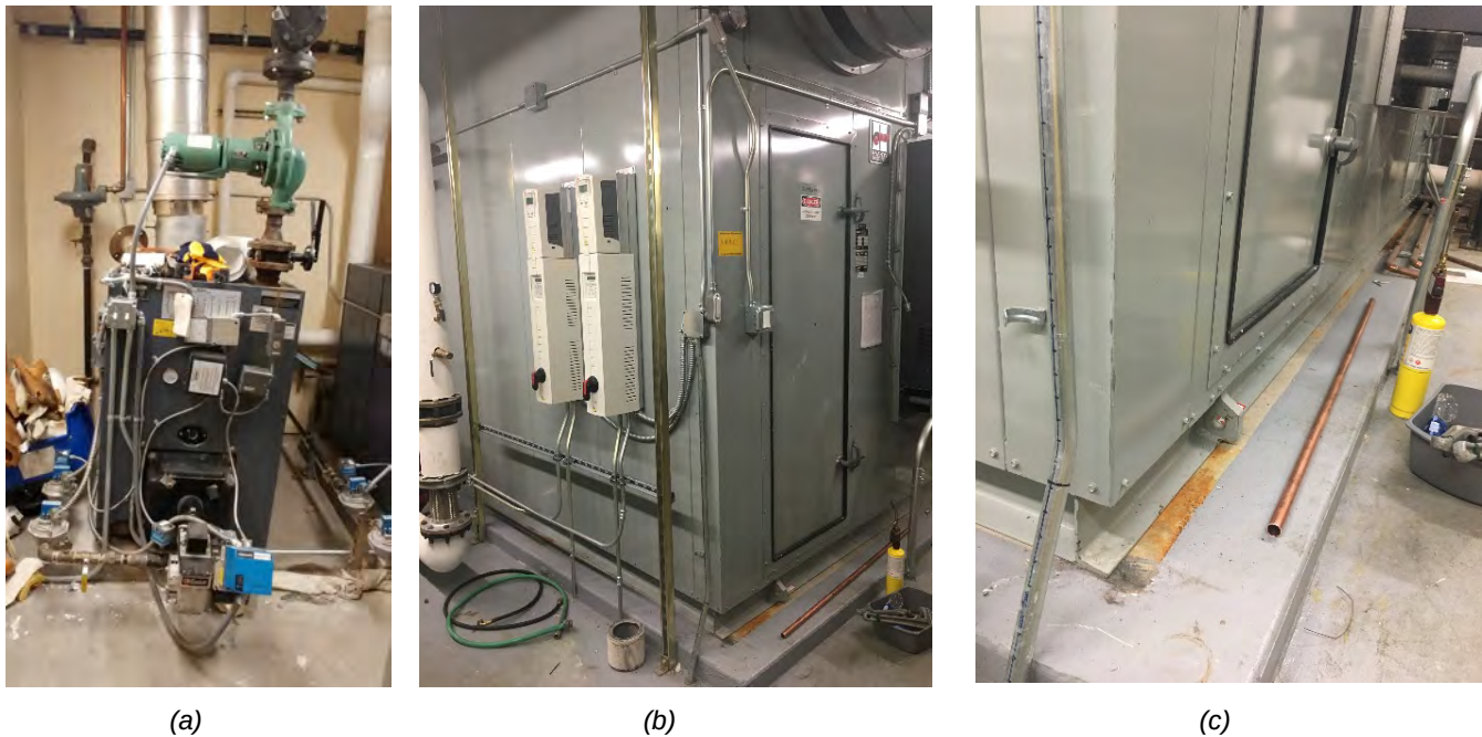
Figure 5.12. (a) Mechanical equipment damage, (b), (c) Mechanical unit sliding for a few inches: fourth floor of a hospital building, Anchorage (photos: (a) Greg Latreille; (b), (c) Wael Hassan).
