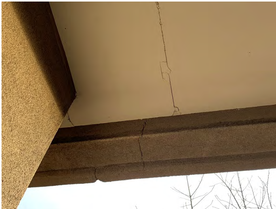
Figure 7.8. Flexural cracking in spandrel concrete in an Anchorage hospital's parking structure. Ceiling-finish cracking here might imply hidden concrete slab damage (photo: Wael Hassan).
