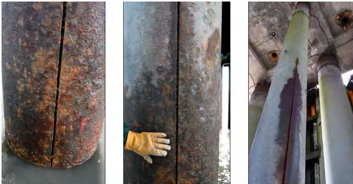
Figure 9.17. Weld failure in vertical seam of wharf pile at Terminal 2 (photos: Port of Alaska).
