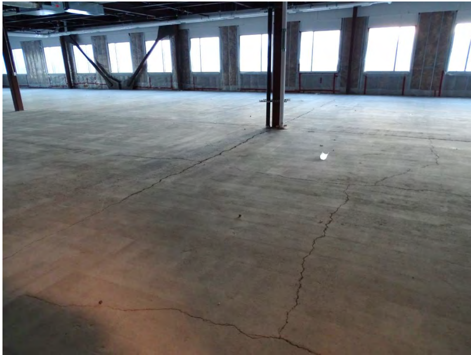
Figure 7.9. Slab cracking viewed from the second floor of Mat-Su Regional MOB 2, attributed by building personnel to the earthquake (photo: Janise Rodgers).
