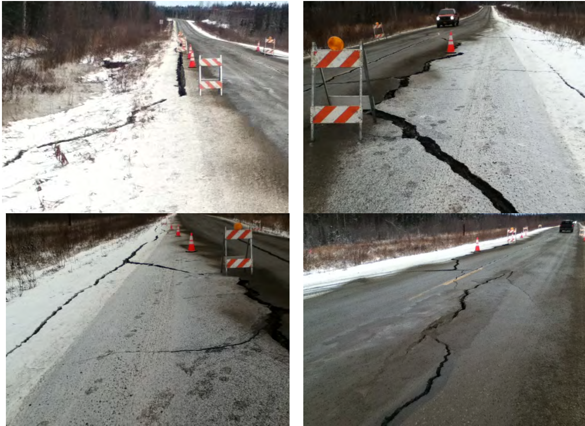
Figure 8.26. Damage to Point Mackenzie Road.
