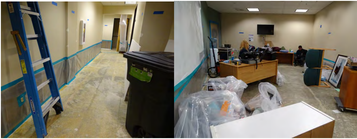
Figure 7.16. Remediation of damage due to water and glycol leaks at Mat-Su Regional MOB 1 on December 11 (photos: Janise Rodgers).
