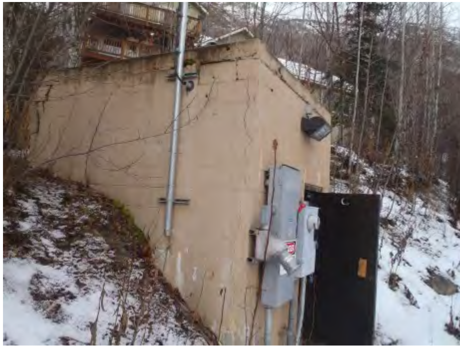
Figure 9.11. CMU damage at the Hyland Crest Booster Station in Eagle River (photo: AWWU).
