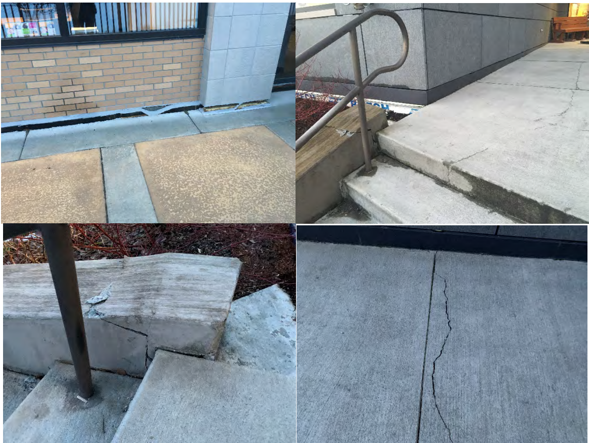
Figure 7.12. Geotechnically related structural damage in a hospital in Anchorage (photos: Wael Hassan).
