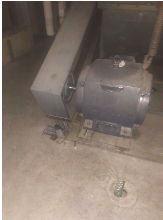
Figure 5.14. Broken nonseismic vibration isolator, Bartlett High School (photo: ASD).
