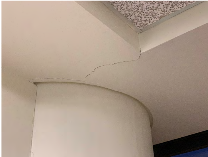
Figure 4.53. Third-floor column-head finish cracks; cracks in gypsum ceilings could potentially indicate hidden floor-diaphragm damage (photo: Wael Hassan).
