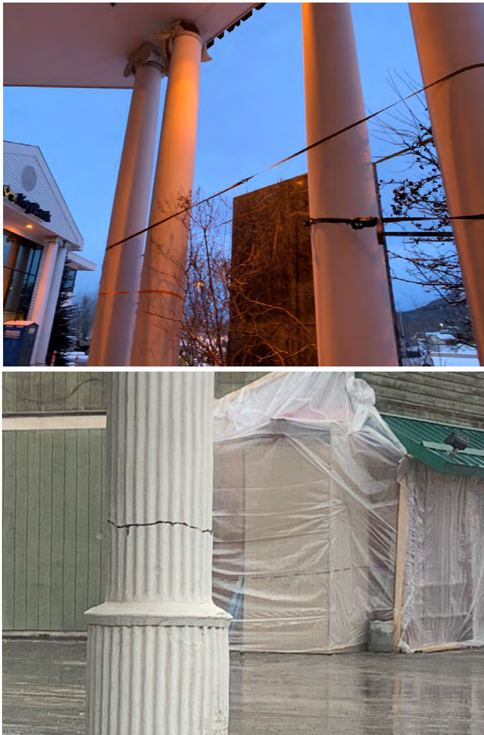
Figure 5.24. Damage in architectural columns at an Eagle River business building (photos: Wael Hassan).
