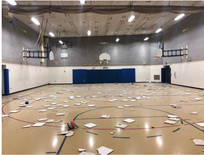
Figure 6.21. Fallen adhered acoustical tiles in gymnasium, Eagle River Elementary (photo: ASD).
