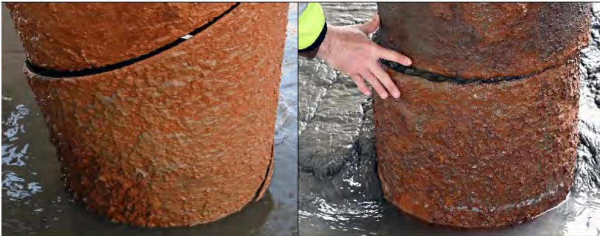
Figure 9.16. Weld failure in spiral seam of wharf pile (photo: Port of Alaska).
