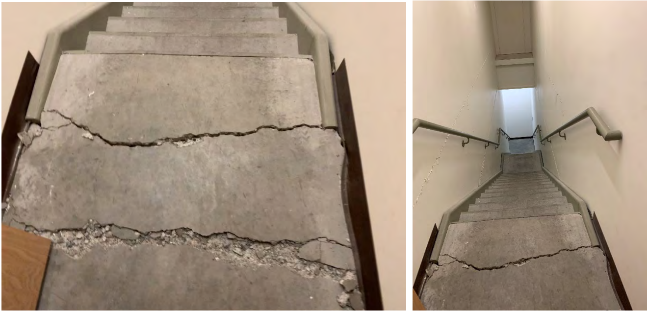
Figure 7.11. Cracking and crushing of concrete at stair flight-landing interface, BBA (photos: Wael Hassan).
