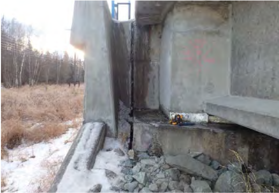
Figure 8.13. Wing wall 1.5-inch displacement for 20 feet (photo: Nick Murray and Ben Still).
