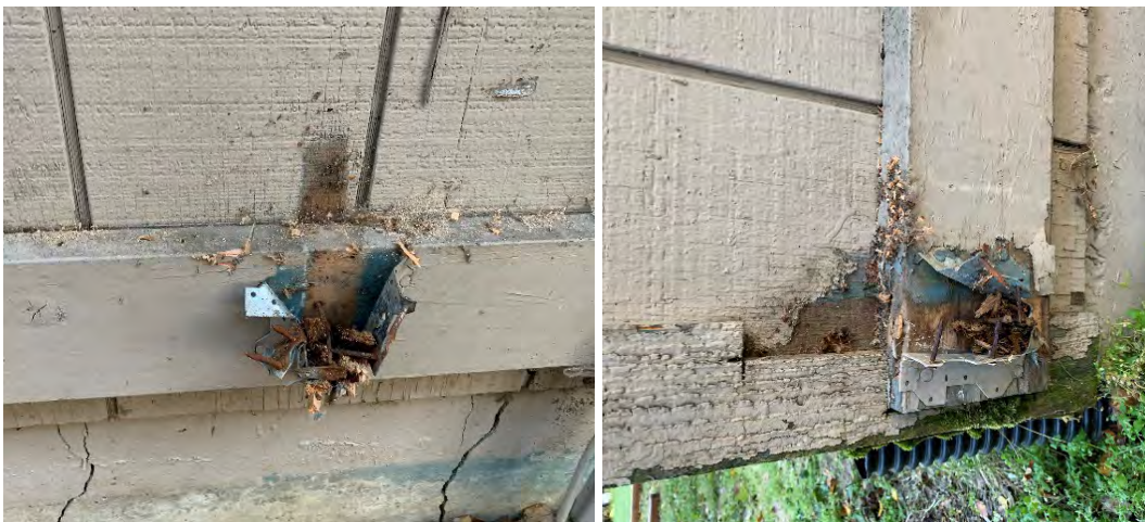
Figure 4.39. Severe shear wall and nailed-connection damage in a residential building in Anchorage (photos: Wael Hassan).
