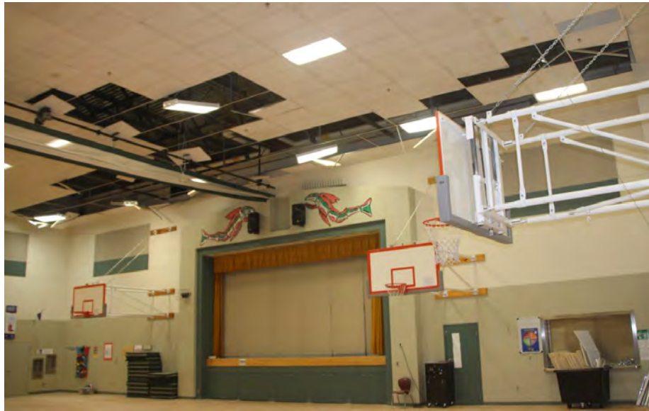
Figure 5.33. Damage to a suspended grid ceiling at Finger Lake Elementary School in Mat-Su (photo: Chris Motter).
