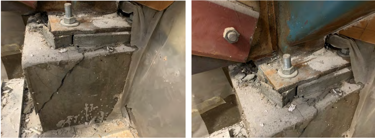
Figure 4.41. Foundation damage and base plate grout pad crushing in several retrofit steel braces in the Anchorage office building. Bolts were loosened by the ground motions on several base plates. No evidence to support soil problems at the area and the damage is believed to be due to retrofit system design errors. (photos: Wael Hassan)
