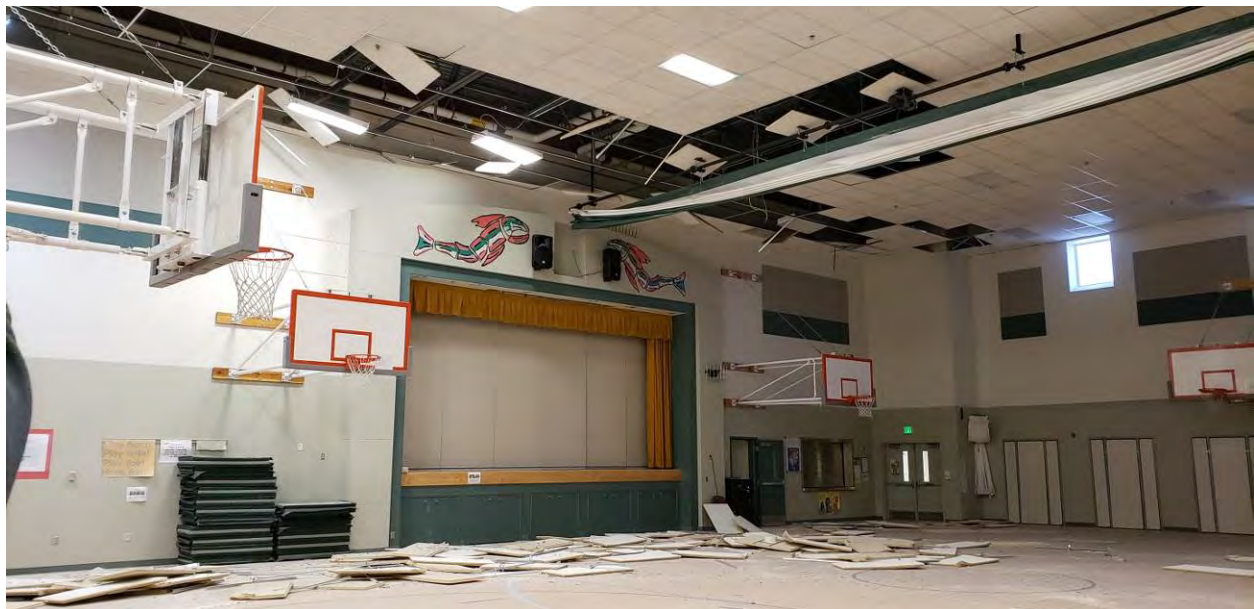
Figure 6.20. Ceiling damage at Knik Elementary; this ceiling had unusually thick and heavy panels (photo: MSBSD).
