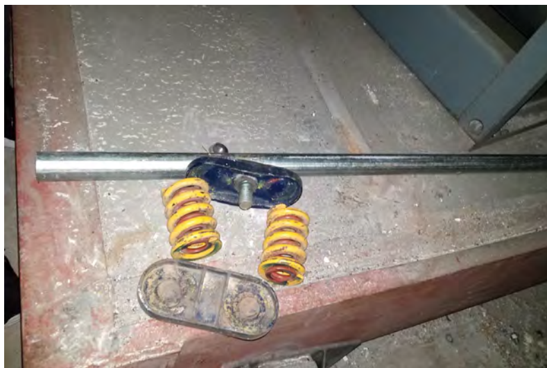
Figure 5.15. Isolator and snubber failures due to improper and undersized anchorage (photos: Randall Williams 2 ).
