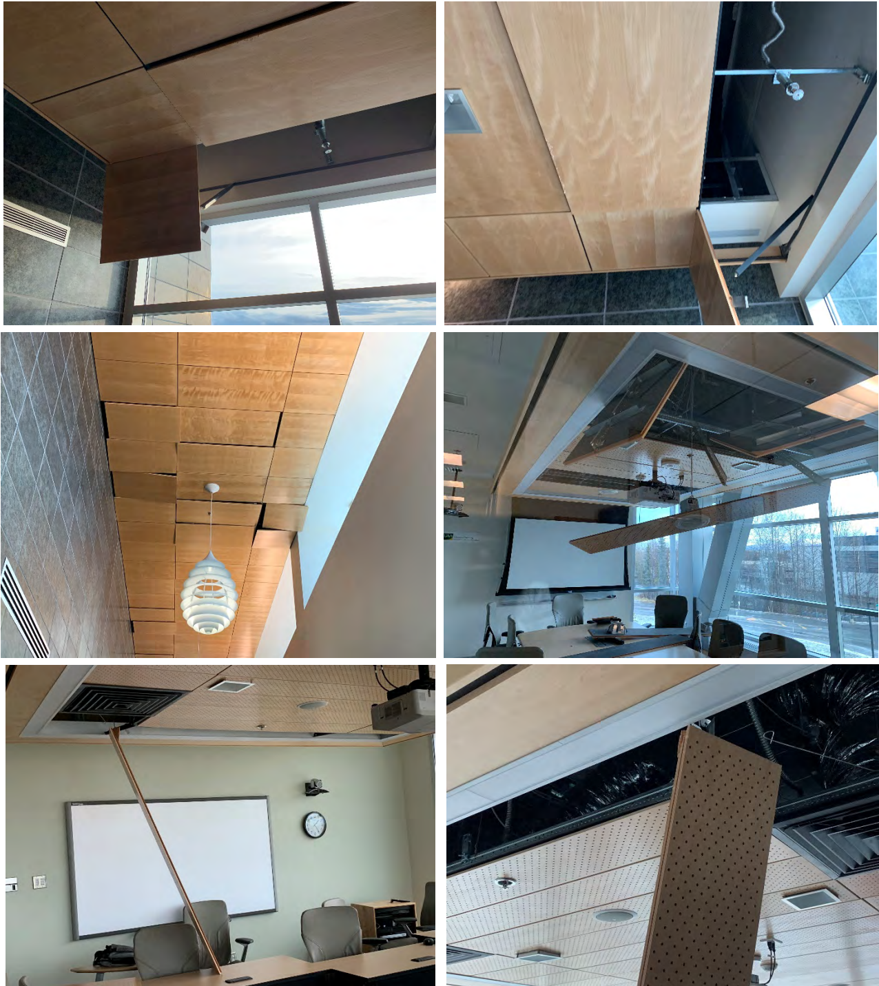
Figure 5.32. The 2015 UAA HSB (PGA 0.21g) ceiling damage. Large, heavy wooden ceiling tiles fell, and the grid failed because of wire snapping; however, in the same building, the acoustic light tiles and grid had minimum damage (photos: Wael Hassan).
