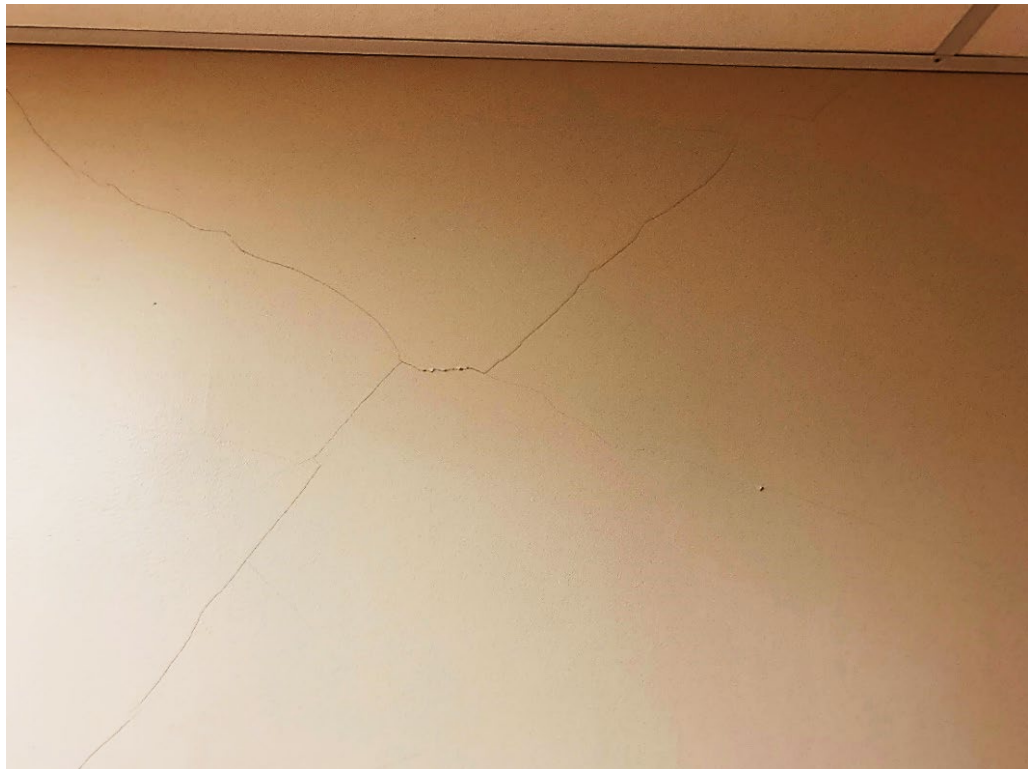
Figure 4.13. Concrete core wall with cross shear cracks in a multistory Anchorage building (photos: Wael Hassan).
