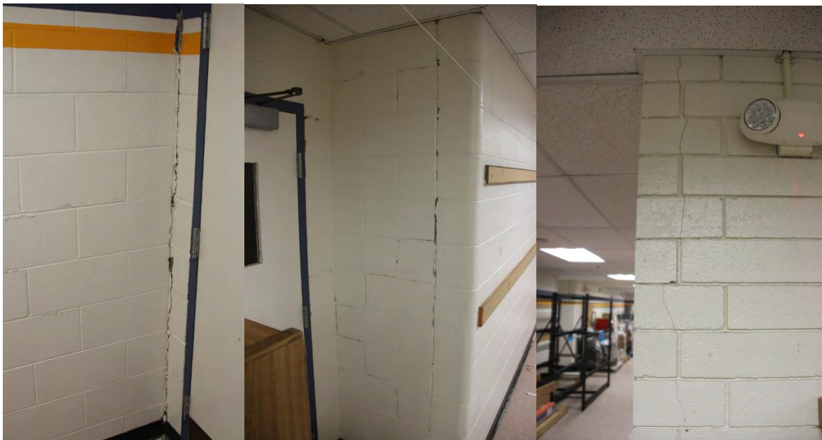
Figure 6.7. Vertical cracking at interface of perpendicularly oriented masonry walls at Eagle River Elementary (photos: Chris Motter).
