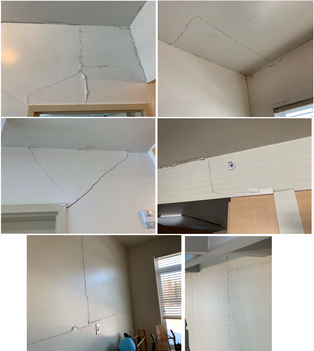
Figure 5.40 Typical partition-wall sheetrock damage in office, hospitality, religious, and educational buildings in Anchorage and Eagle River (photos: Wael Hassan).
