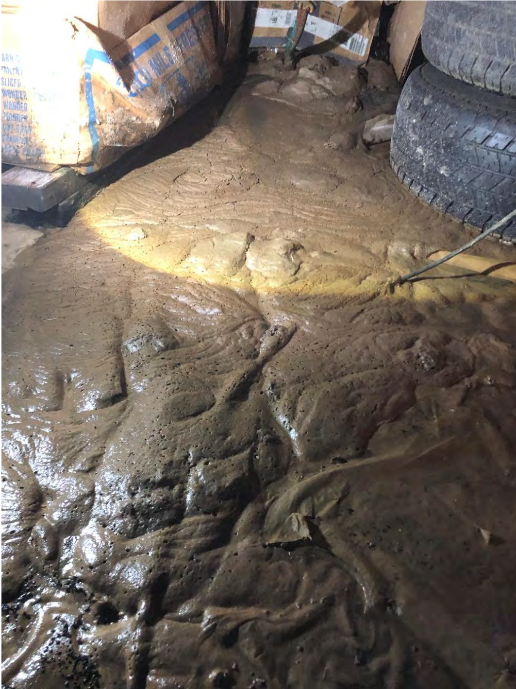
Figure 3.1. Liquefaction sand ejecta in residential crawl space (photo: Howard Weston).
