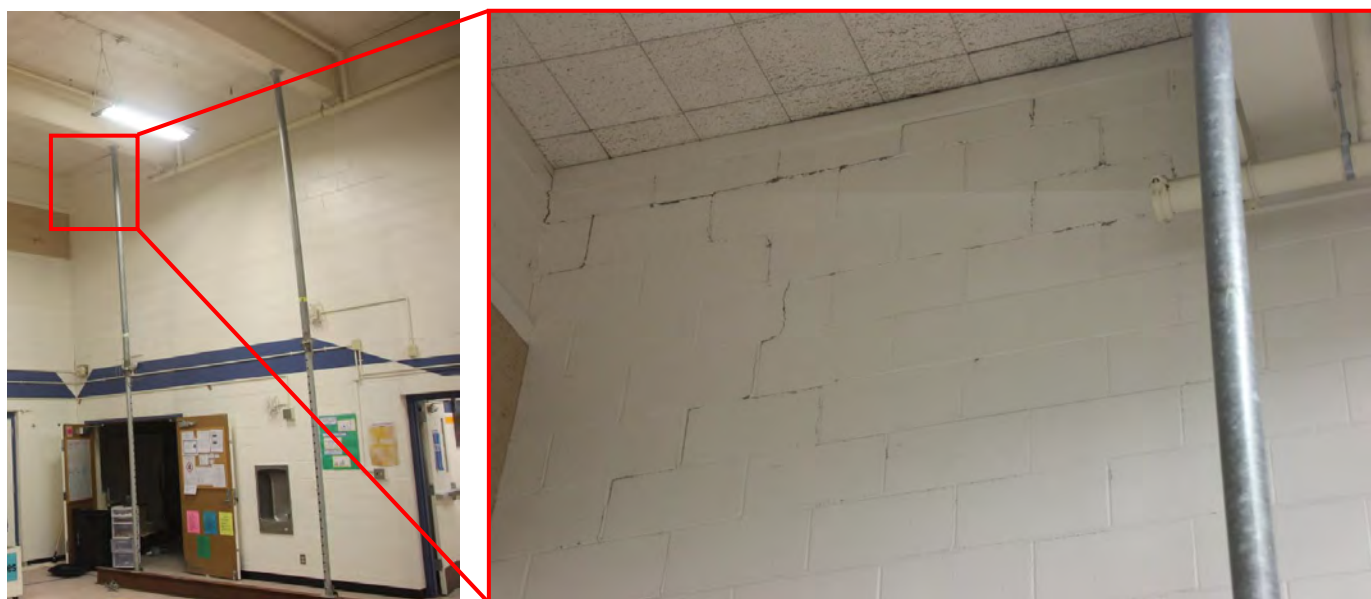
Figure 6.8. Cracking at upper corner of masonry wall at Eagle River Elementary; note vertical shoring due to failed roof-wall connections (photo: Chris Motter).
