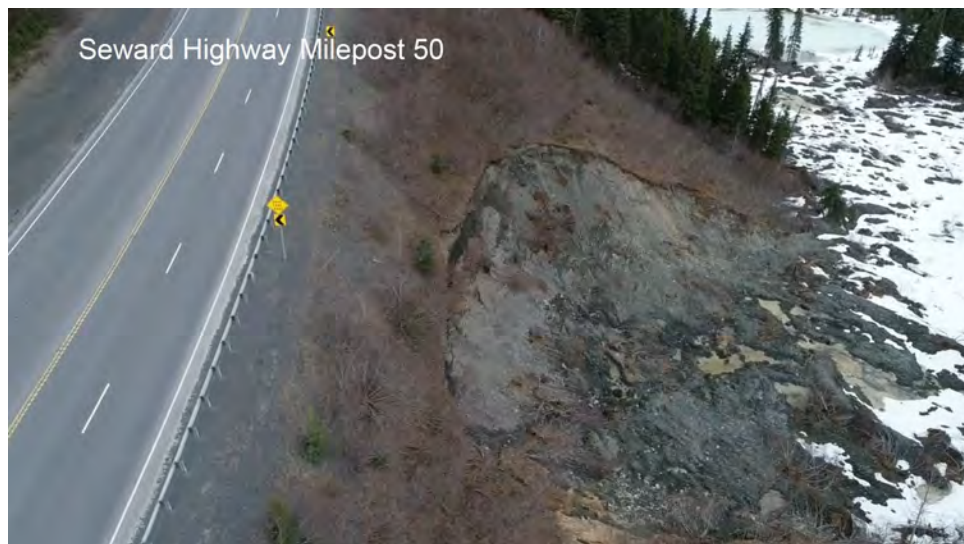
Figure 8.18. Seward Highway milepost 50 damage (source: Thornley, 2019).
