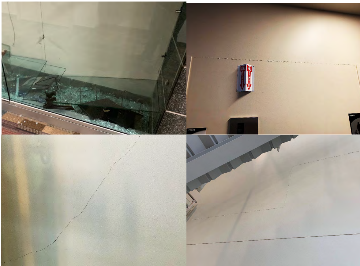
Figure 4.62. EIB, UAA, non-structural sheetrock damage throughout the building and a glass cabinet damage in the fourth floor (photos: Wael Hassan).
