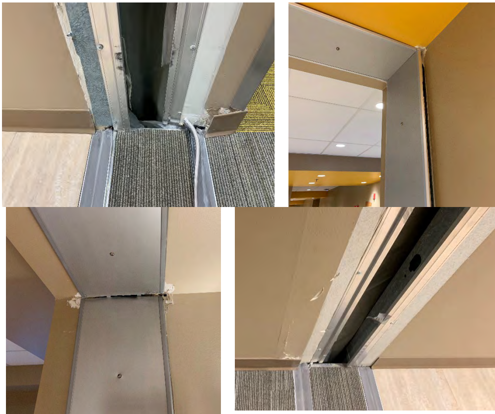
Figure 7.6. Examples of seismic joint damage at an Anchorage hospital (photos: Wael Hassan).
