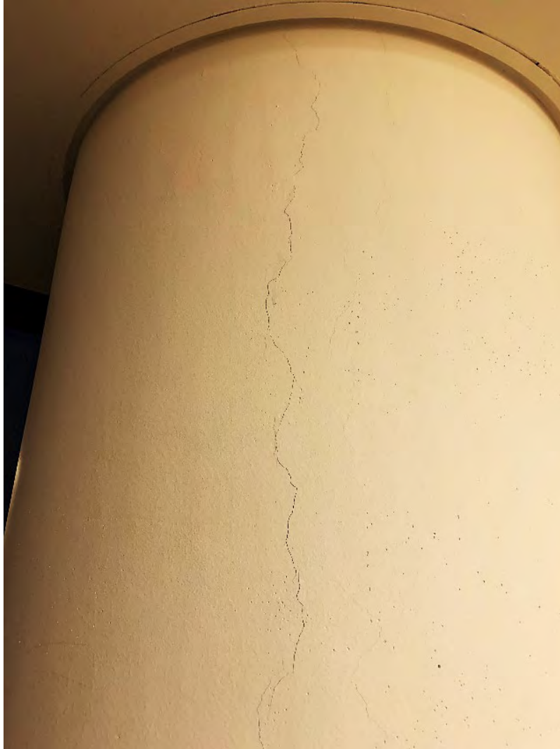
Figure 4.16. Typical splitting crack in exterior-column cover. Most exterior and corner columns on levels one through three exhibited such cracks with variable sizes (photo: Wael Hassan).
