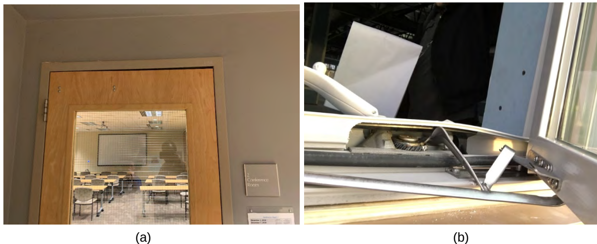
Figure 7.29. Examples of (a) door jamming and (b) window system failure in Anchorage hospitals (photos: Wael Hassan).
