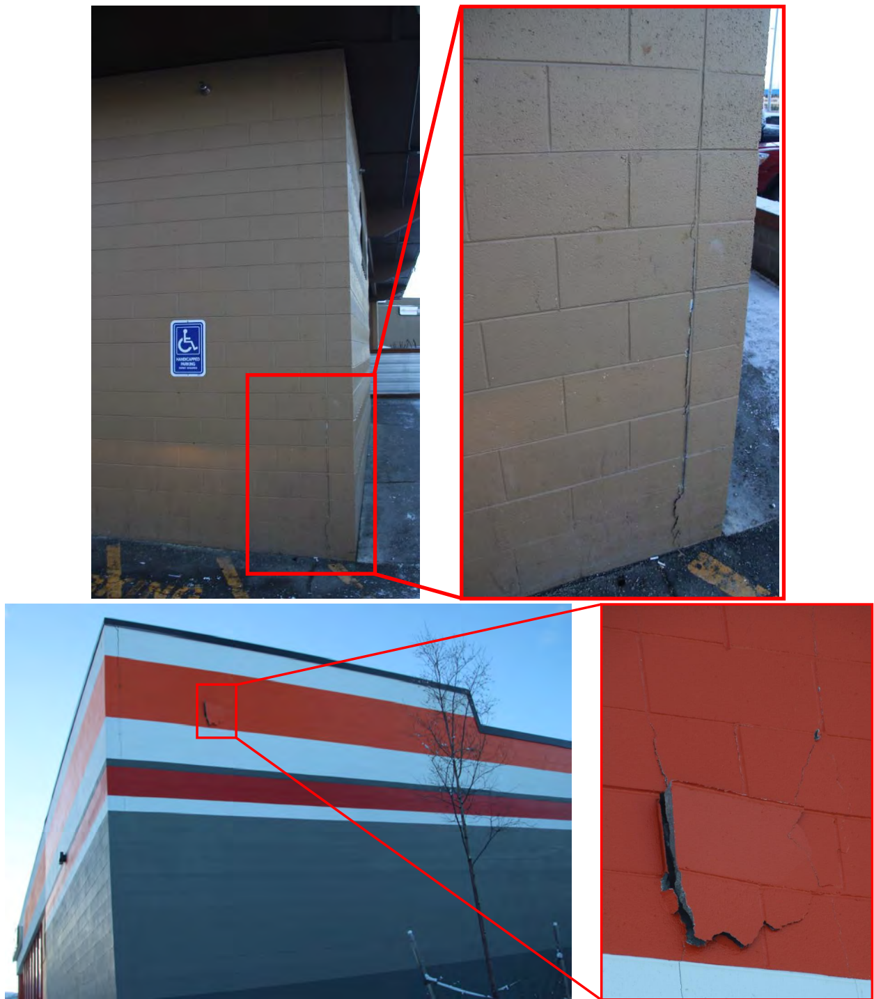
Figure 4.28. Damage in masonry walls, including damage at interfaces of perpendicularly oriented walls (photos: Chris Motter).
