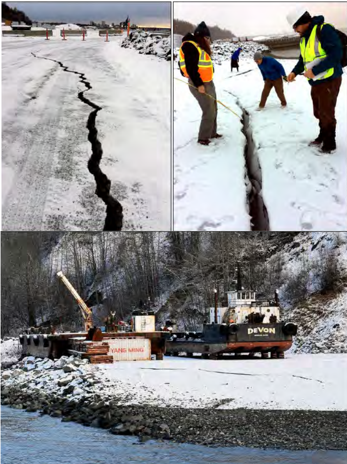
Figure 9.23. A barge and tugboat remain on their blocks despite being in close proximity to slope failures (photos: Port of Alaska).
