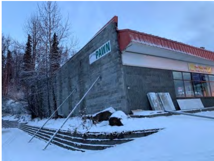
Figure 4.21.a. CMU wall-wall and wall-floor connection failure and out-of-plane deformation of a CMU wall, leading to incipient collapse (photo: Wael Hassan).
