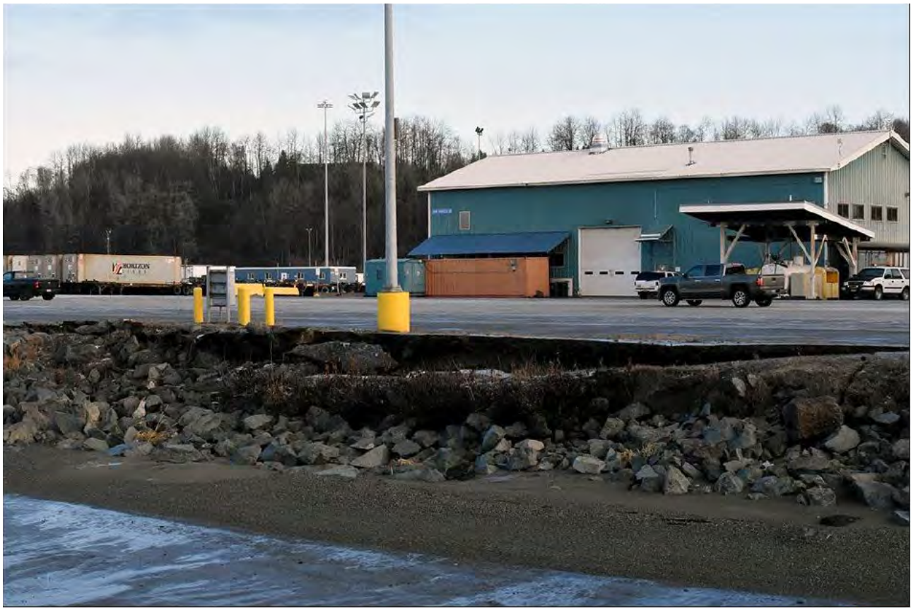
Figure 9.20. Shore failure near Terminal 1 (photo: Port of Alaska).
