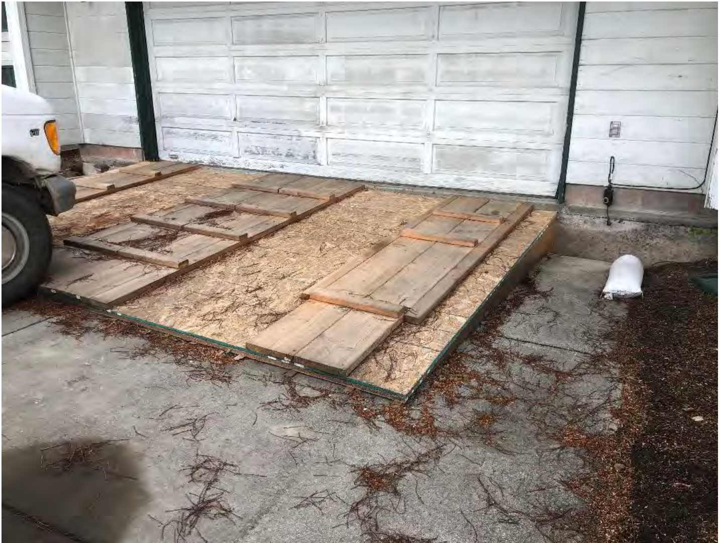
Figure 3.5. Driveway settlement at a residential driveway (photo: Howard Weston).
