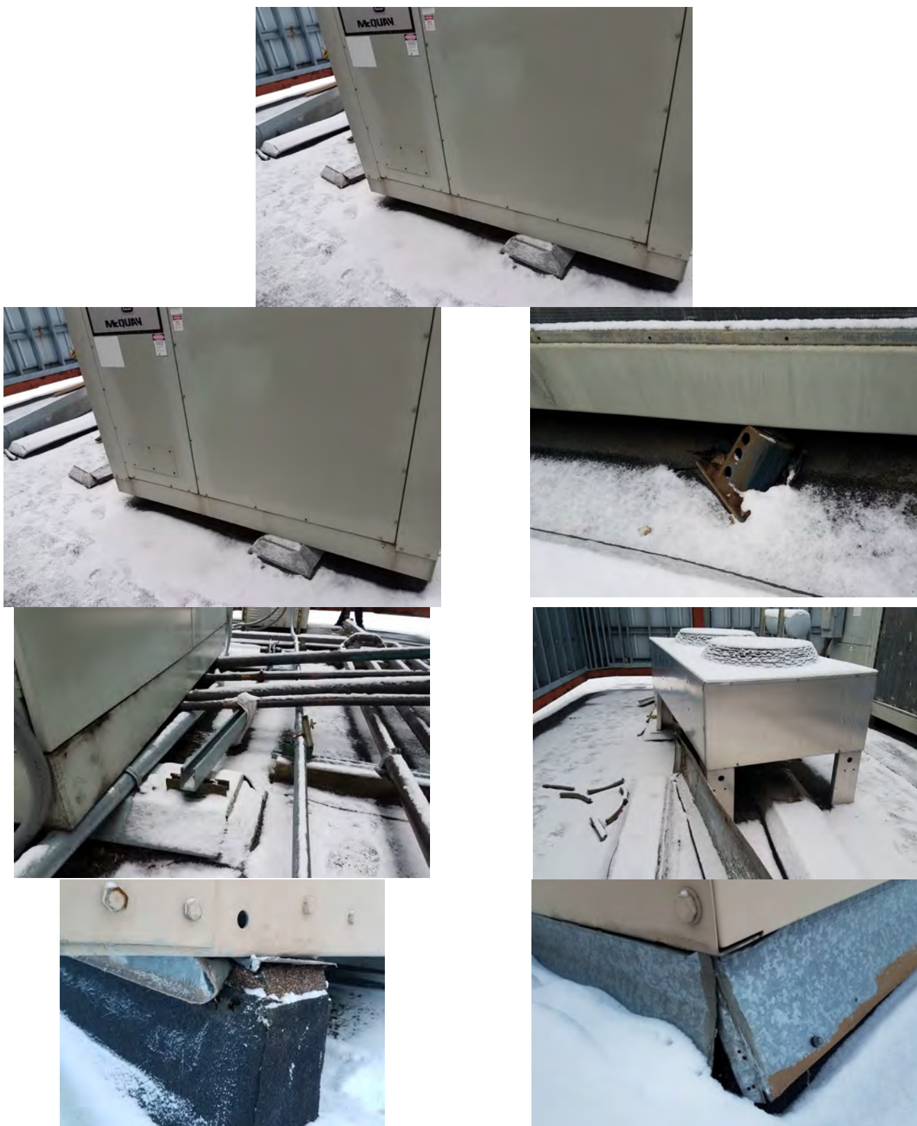
Figure 5.16. Mechanical-equipment sliding and anchorage failure on roof (photos: Randall Williams 2 ).
