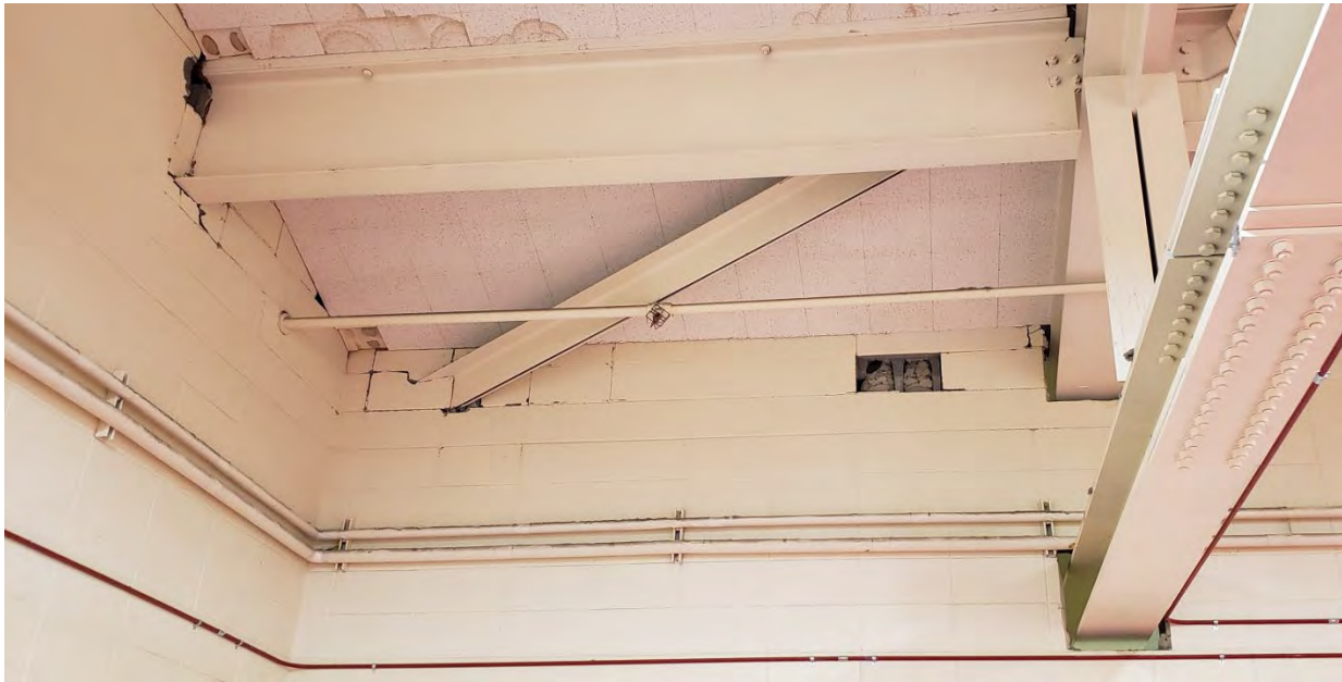
Figure 6.3. CMU block at top of wall cracked and loosened because of differential motion of steel roof framing, Houston Middle School. Loose blocks pose a falling hazard to those below (photo: MSBSD).
