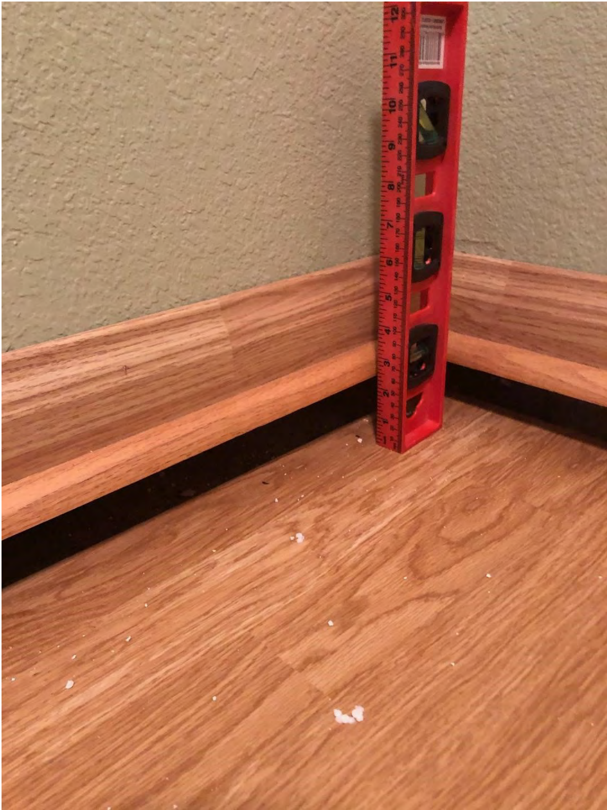
Figure 3.3. Slab on grade liquefaction-induced settlement of 6 cm (photo: Howard Weston).
