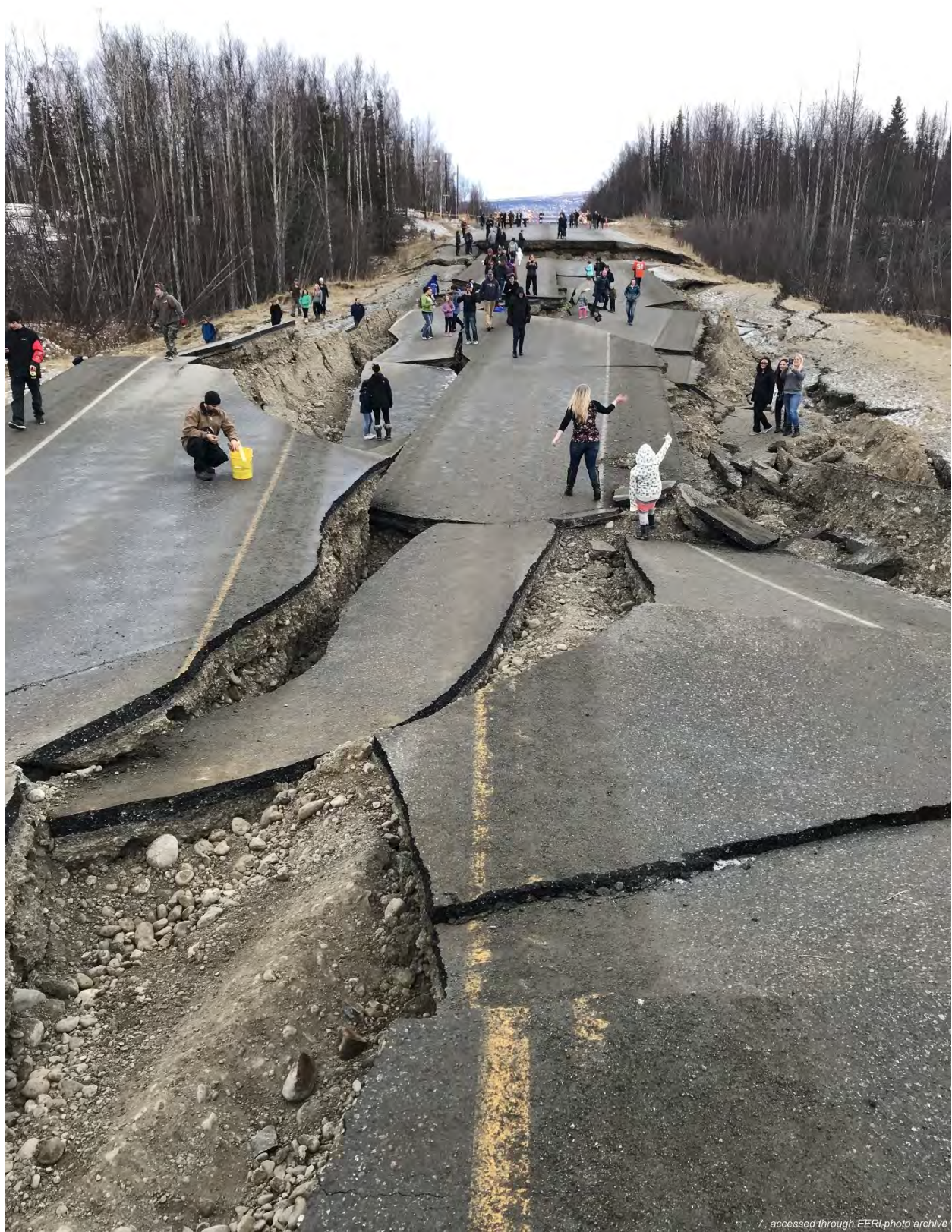
Figure 3.6. Vine Road failure (photo: Earthquake Engineering Research Institute (EERI) Clearinghouse).
