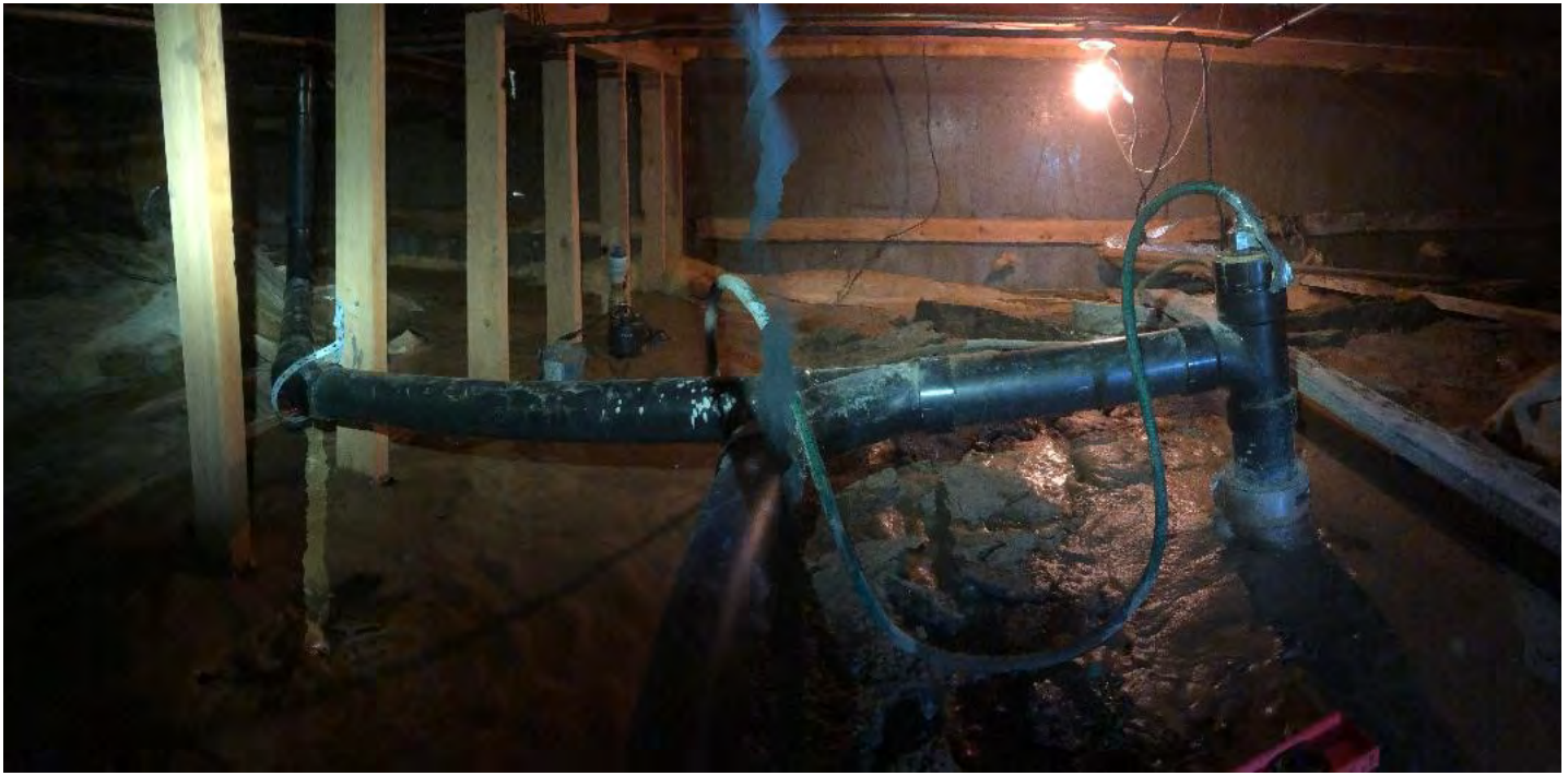
Figure 3.4. Displaced residential sewer service (photo: Howard Weston).
