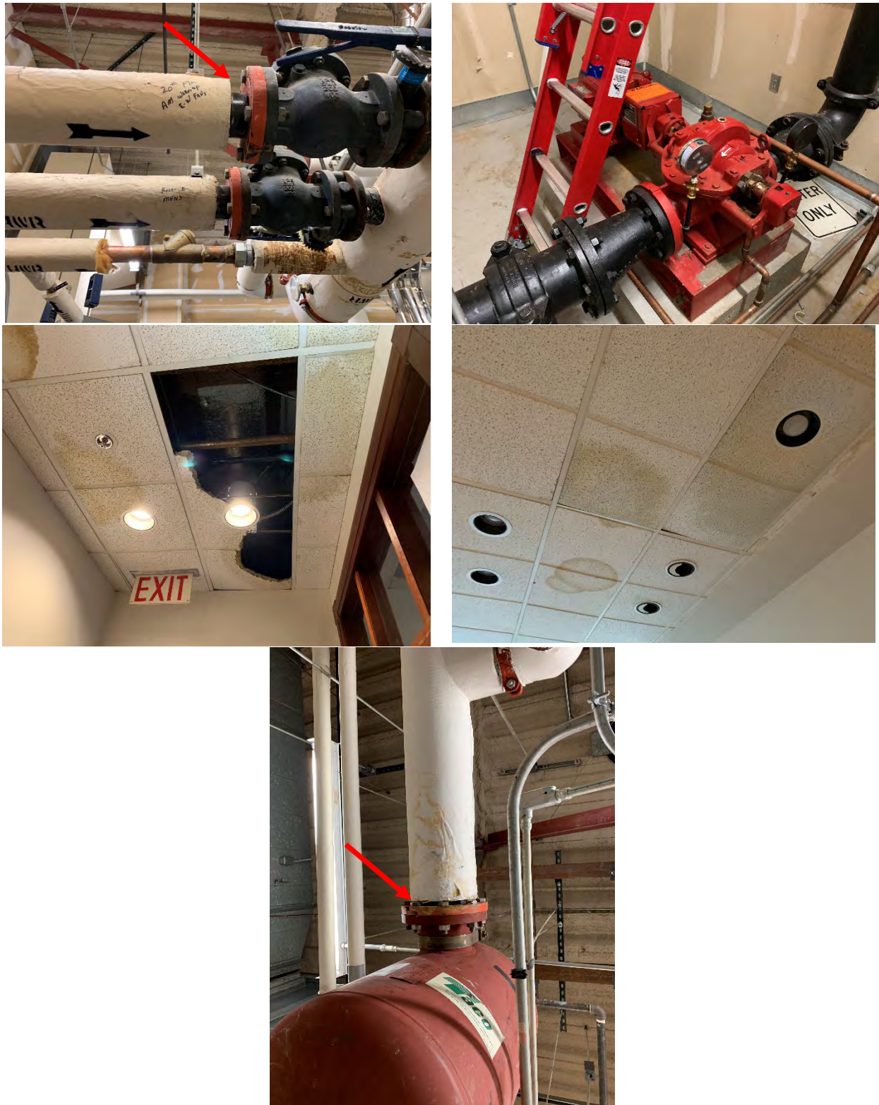
Figure 4.50. Mechanical-room piping failure and water flooding at Atwood Building (photos: Wael Hassan).
