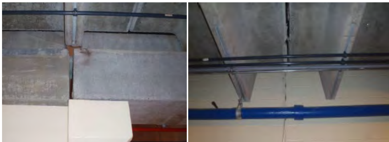
Figure 9.10. Structural damage at Eklutna Water Treatment Plant (photos: AWWU).
