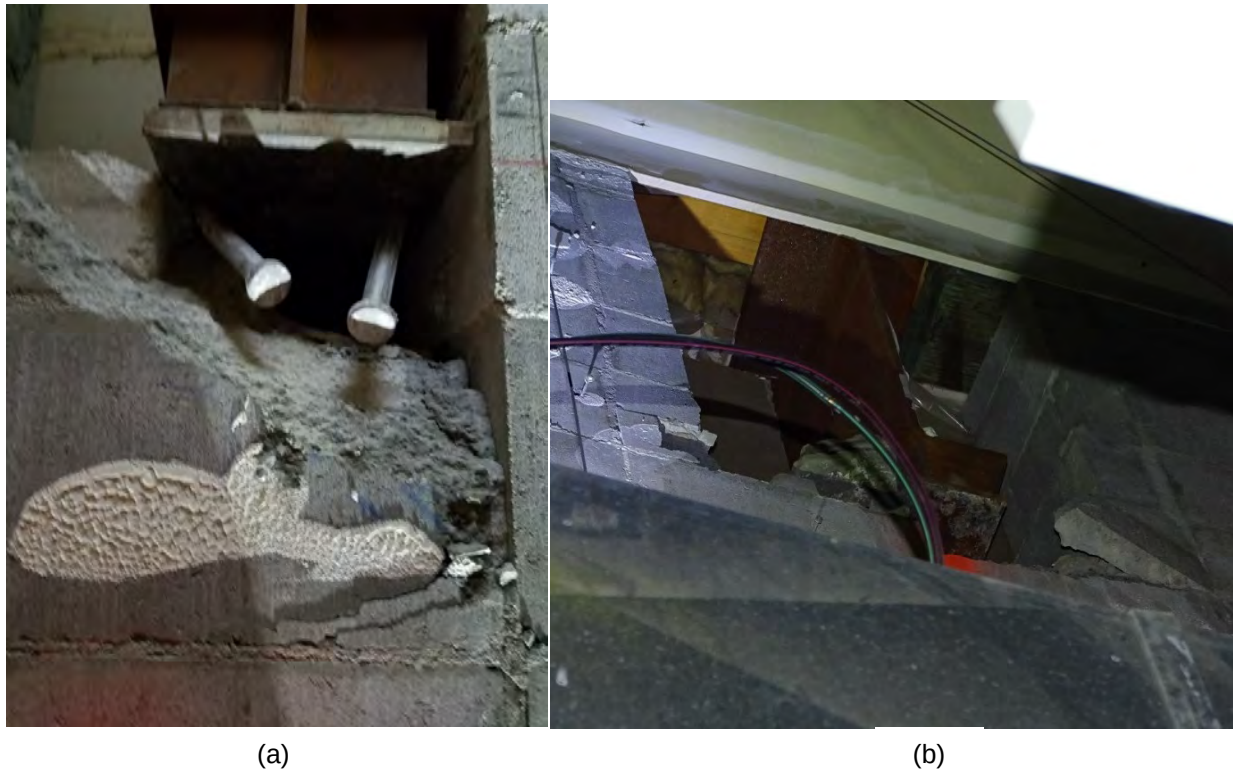
Figure 6.2. Failed connection between a steel roof girder and a CMU wall at Houston Middle School: (a) second story of classroom wing (photo: Bill Noyes) and (b) similar failed connection (photo: Janise Rodgers).
