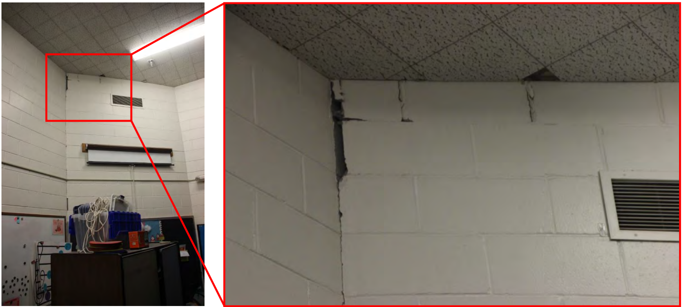
Figure 6.5. Damage to masonry walls at Eagle River Elementary (photo: Chris Motter).
