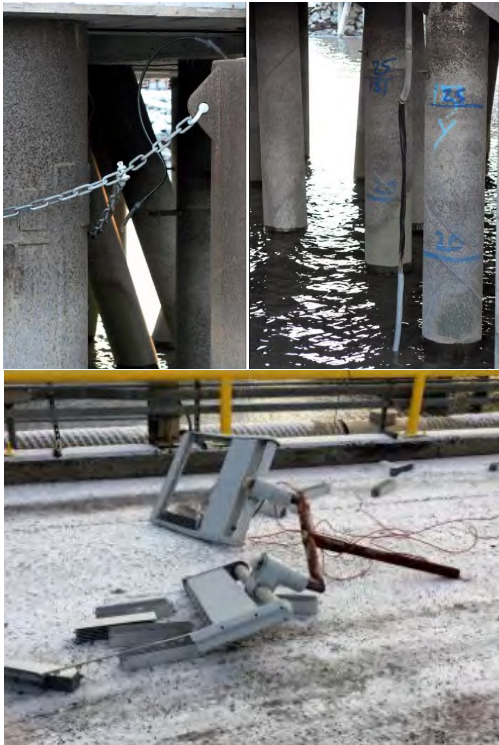
Figure 9.19. Nonstructural damage to dock lights, cameras, and connections and wires of cathodic protection systems (photos: Port of Alaska).
