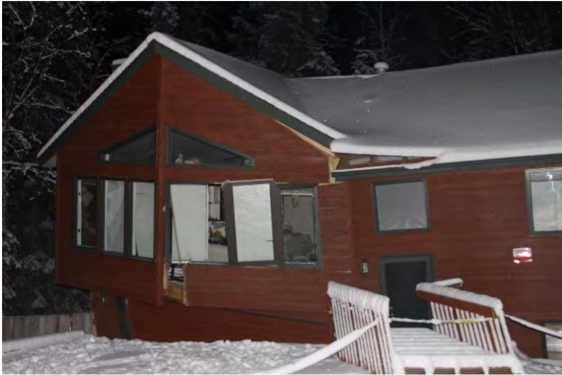
Figure 4.38.a. Residential building damage in Eagle River (photos: Chris Motter).
