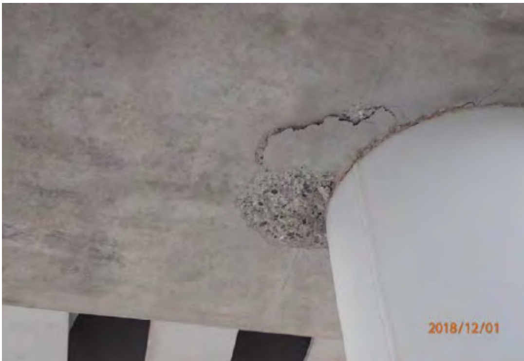
Figure 8.10. Spalling at pile pier cap (photo: Sara Manning and Fred Paulsen).
