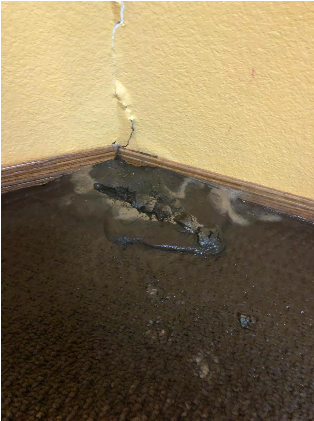
Figure 3.2. Slab on grade liquefaction ejecta (photo: Howard Weston).
