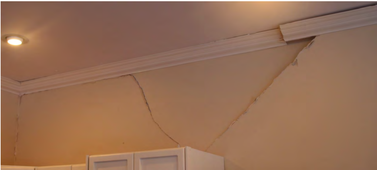
Figure 4.34.b. Example of inside damage to a residential building in Mat-Su (photos: Chris Motter).
