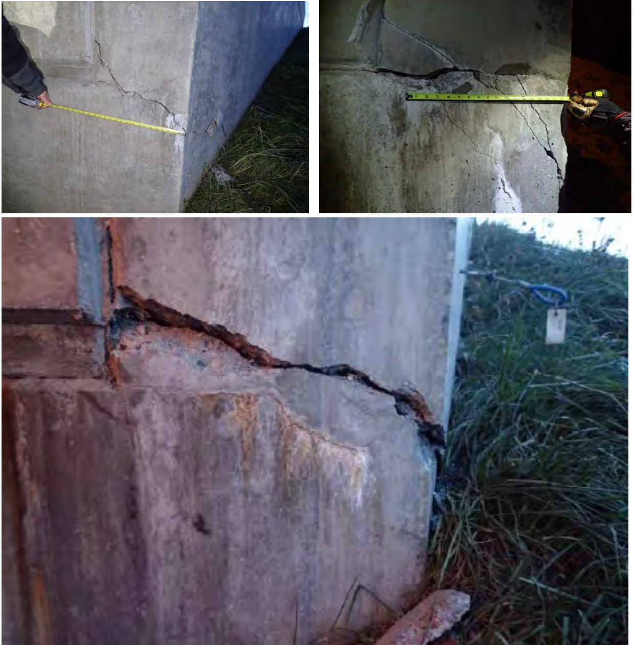
Figure 8.7. Hider wall cracks (photos: Nick Murray and Ben Still).
