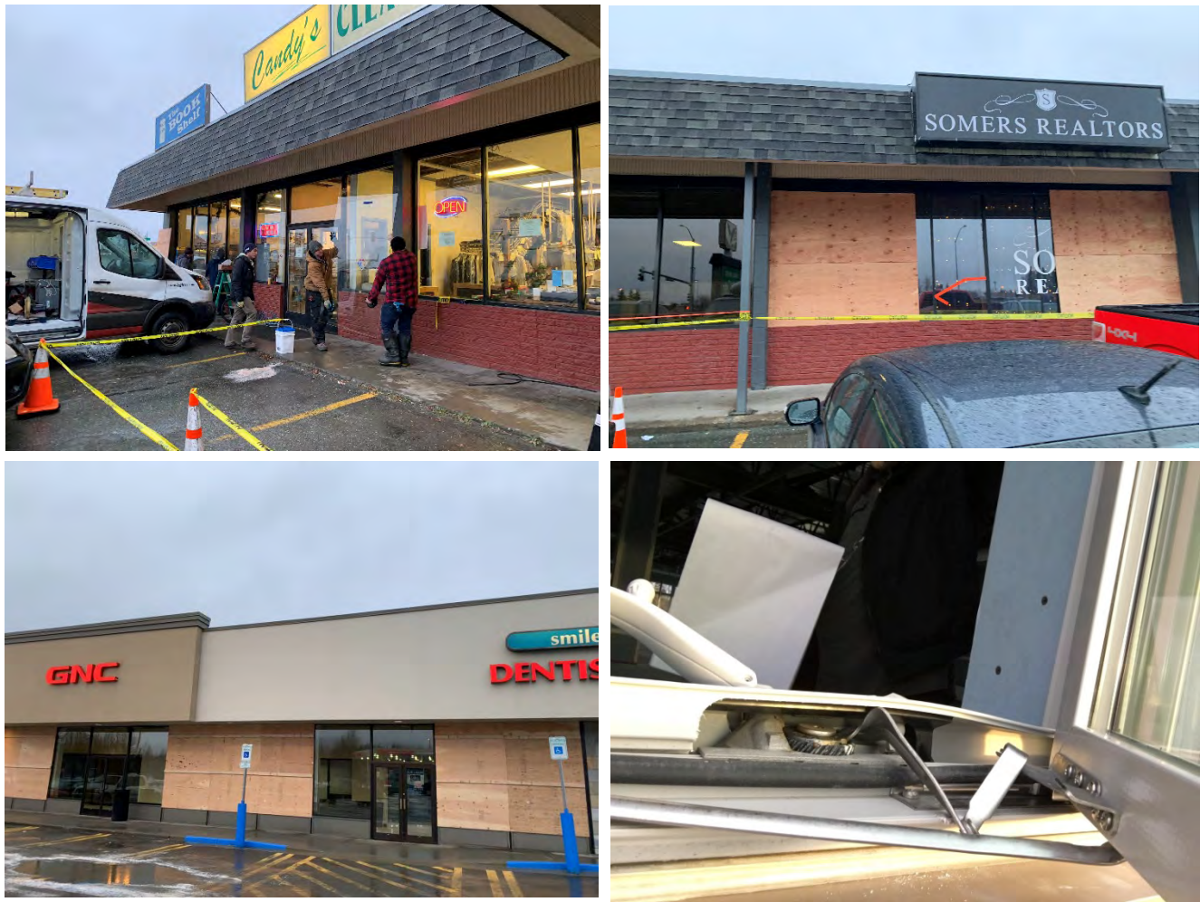
Figure 5.26. Damage to windows at retail and commercial buildings in Eagle River and a hospital in Anchorage (bottom right) (photos: Wael Hassan).
