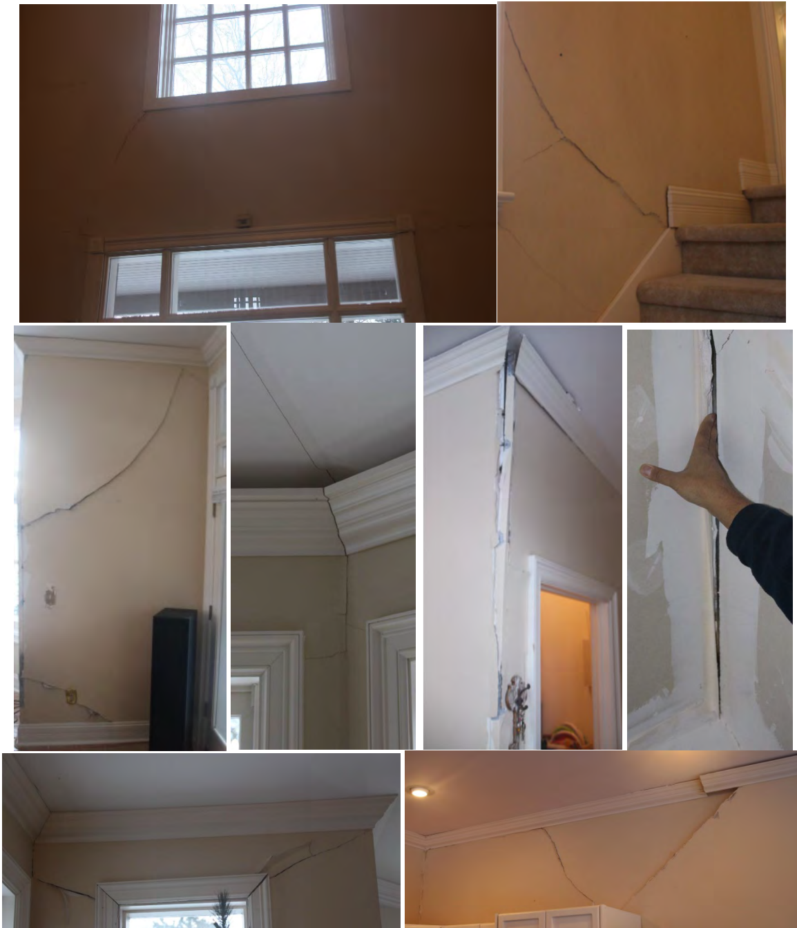
Figure 5.37. Wall damage in a house in Mat-Su near Finger Lake (photos: Chris Motter).
