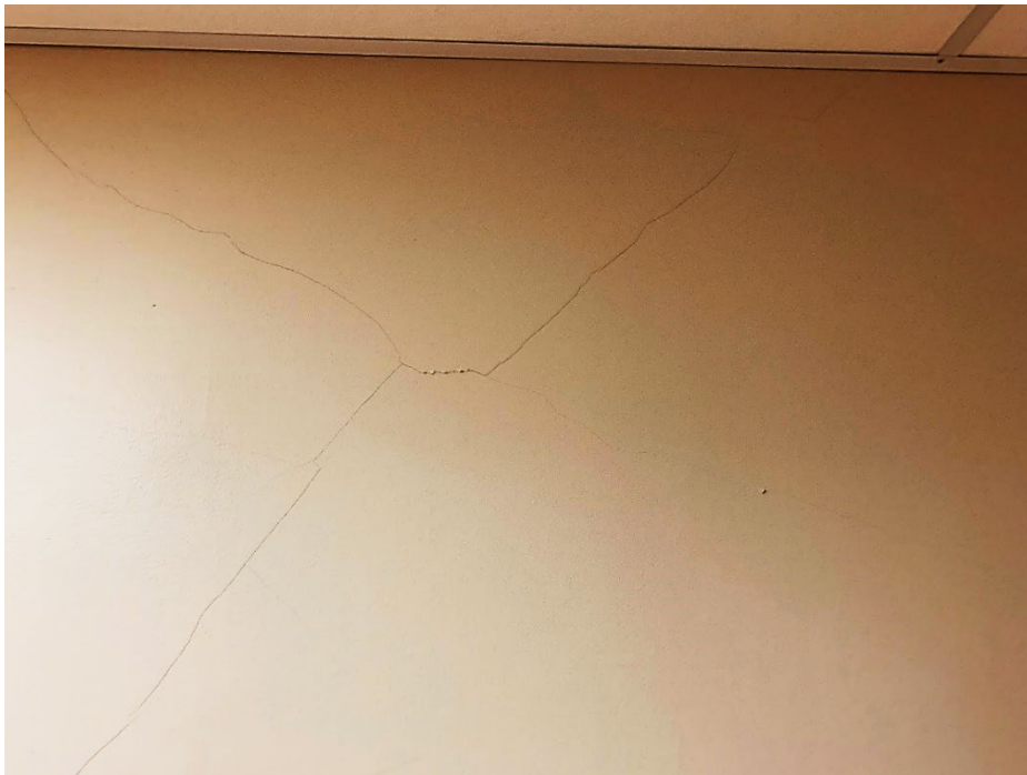
Figure 7.3. Concrete shear wall cross-shaped shear cracks in the main building of an Anchorage hospital (photo: Wael Hassan).
