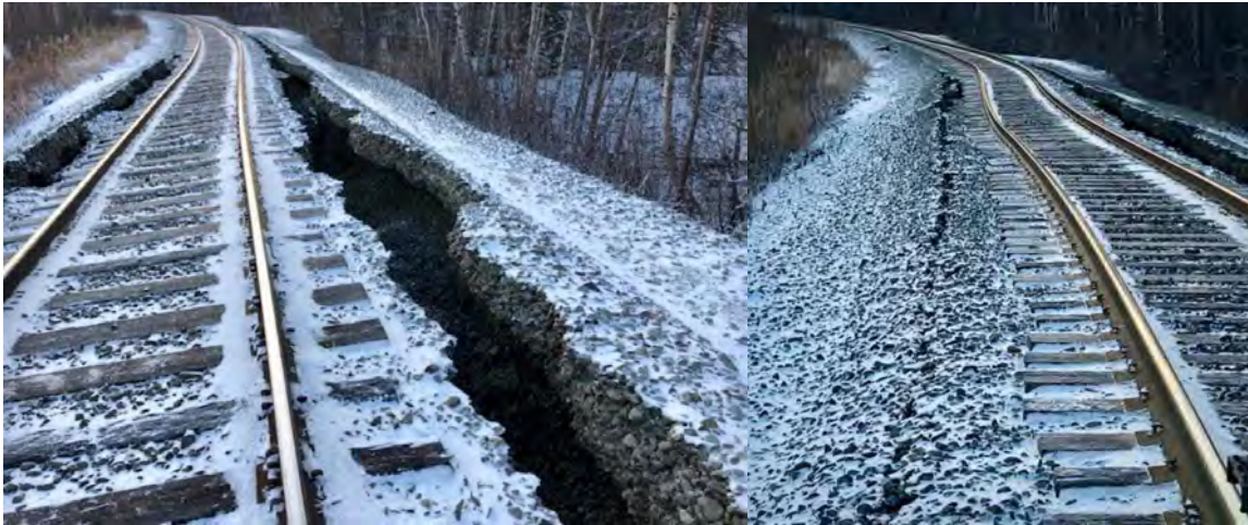
Figure 9.14. Damage to Alaska Railroad (photo: Associated Press, 2018).
