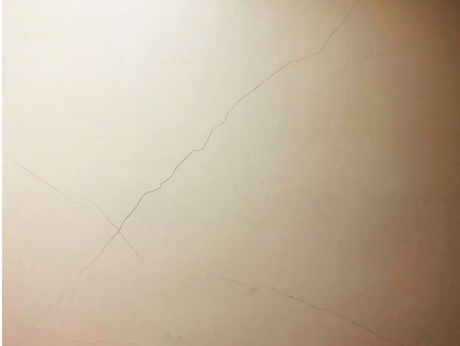
Figure 7.2. Concrete core wall cross-shaped shear cracks in main building of an Anchorage hospital. These cracks are sample of many similar cracks at different concrete shear walls at level 1 of the hospital (photo: Wael Hassan).
