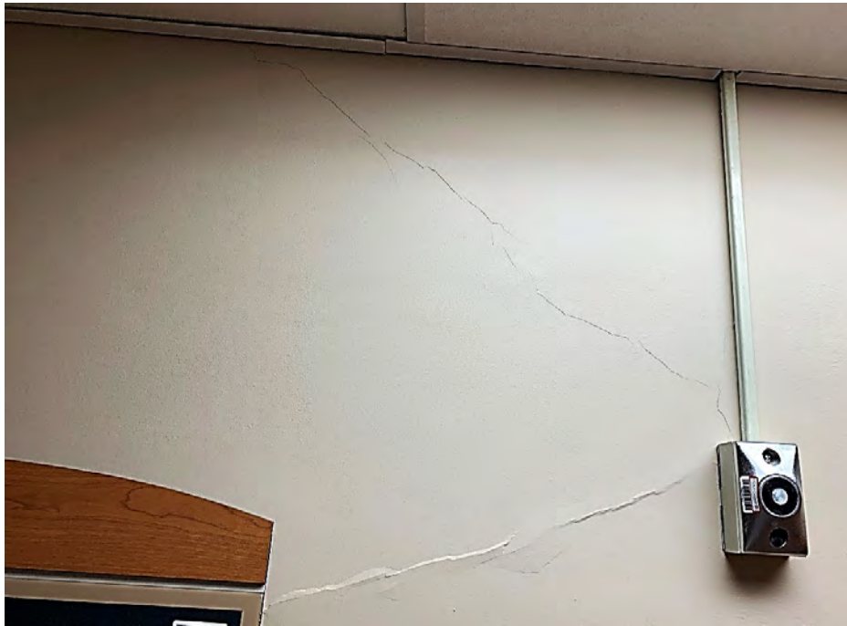
Figure 7.5. Concrete core wall diagonal shear cracks in the main building of an Anchorage hospital (photo: Wael Hassan).
