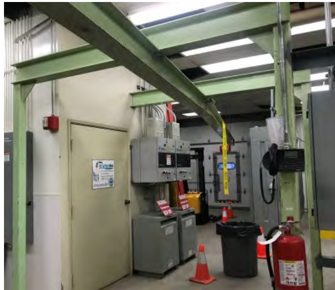
Figure 9.12. Failure in overhead crane beam at Girdwood Wastewater Treatment Facility (photo: AWWU).
