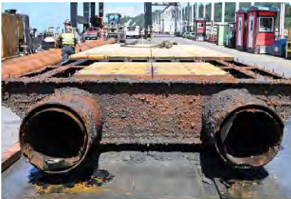
Figure 9.18. Fender pile failures and dock repairs (photo: Port of Alaska).
