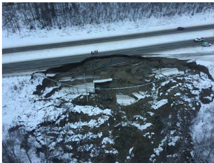
Figure 8.19. Damage to Glenn Highway at Mirror Lake (source: Thornley, 2019).
