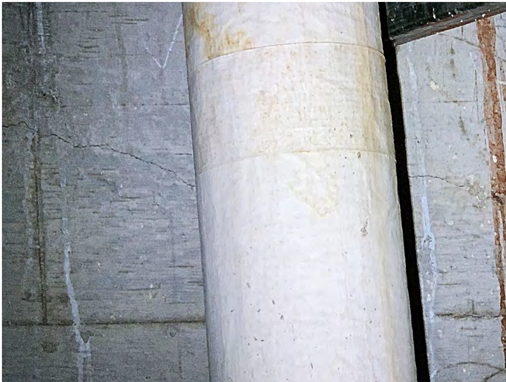
Figure 7.4. Minor concrete core wall diagonal shear crack in the main building of an Anchorage hospital; photos were taken inside the elevator shaft (photos: Wael Hassan).
