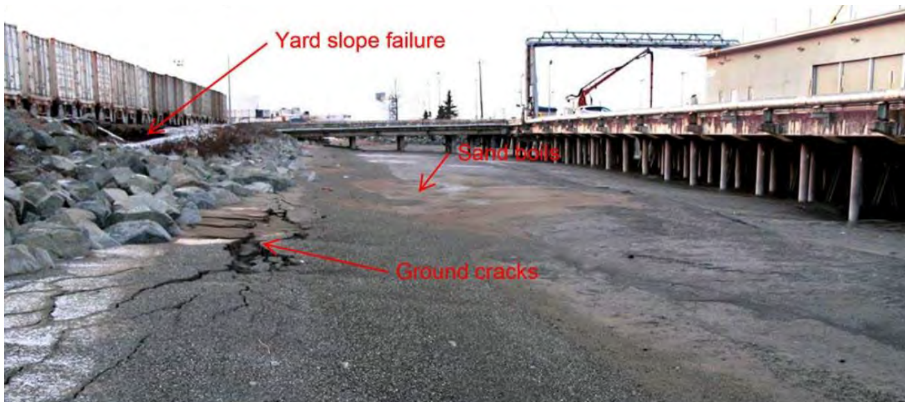
Figure 9.21. Yard slope failure and liquefaction moved shore (photo: Port of Alaska).
