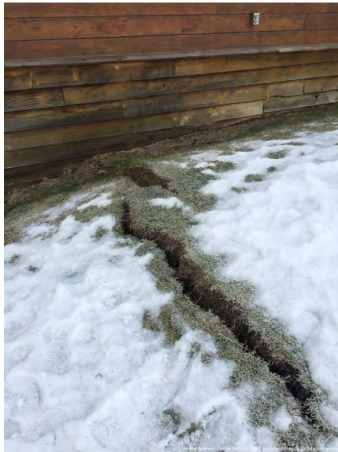
Figure 3.7. Anthropogenic fill failure (photo: EERI Clearinghouse).
