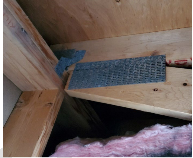
Item F: Truss plate not extending high enough at bearing location (beyond middle depth of the top chord at a minimum)
