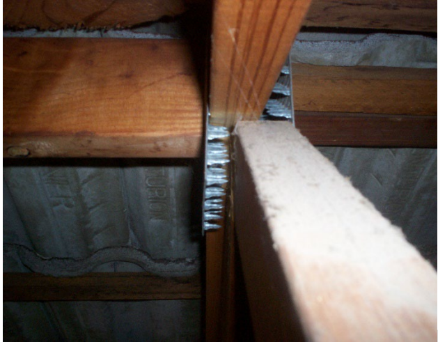
Item A: Incomplete plate connection.
