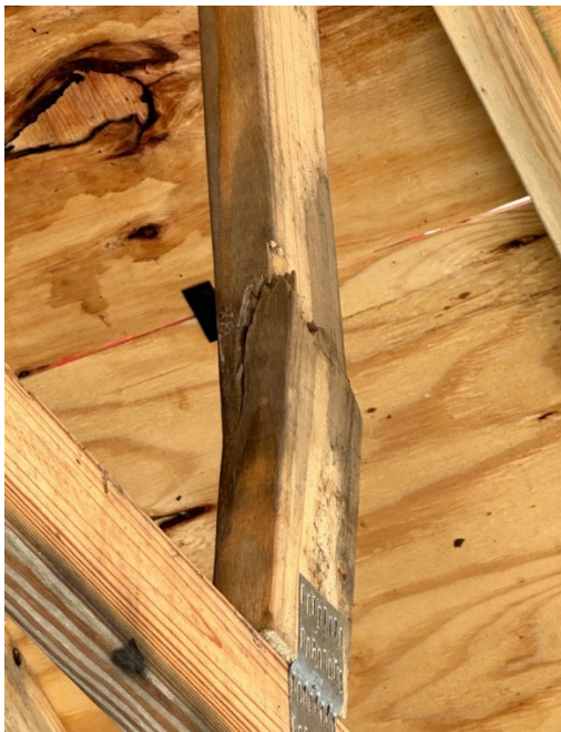
Item C: Web chord broken (likely during construction).
