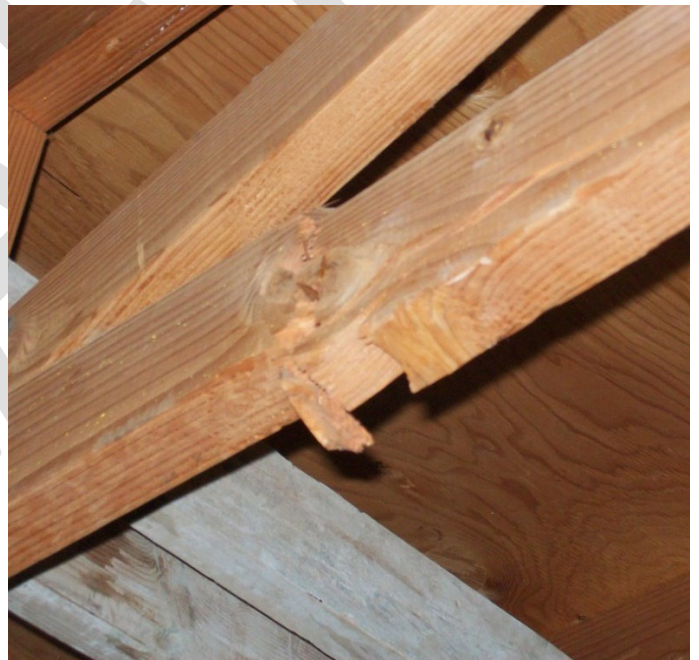
Item D: Bottom chord failure at large knot.
