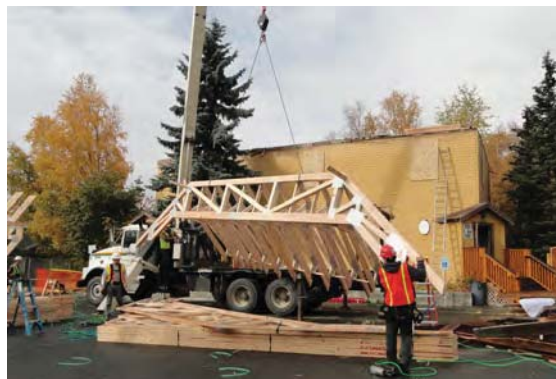
The Historic Preservation Project Fund was recently used by the AHPC to support the replacement of the Pioneer Schoolhouse Roof.
