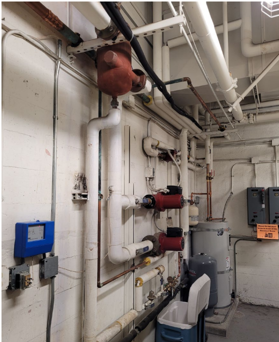
Figure 6 Water heater and pumps to remain
