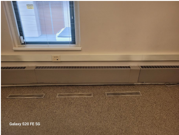
Figure 8 Baseboard and floor grilles
