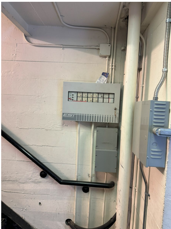
Figure 13 Existing FACP in stairwell
