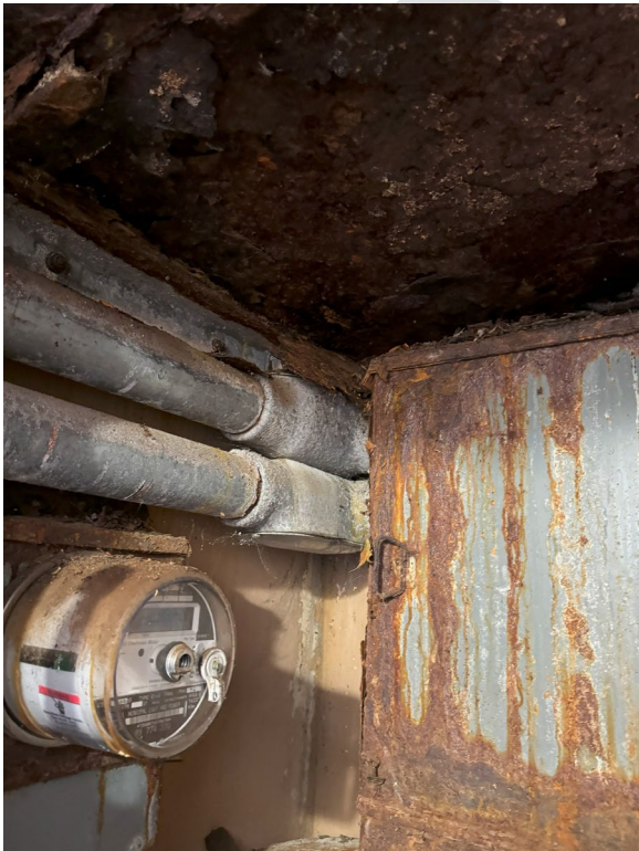
Figure 11 Exterior electrical service equipment
