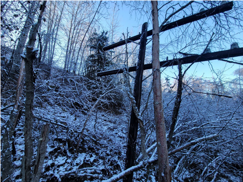
Figure 3. Pole close-up with insulators.
