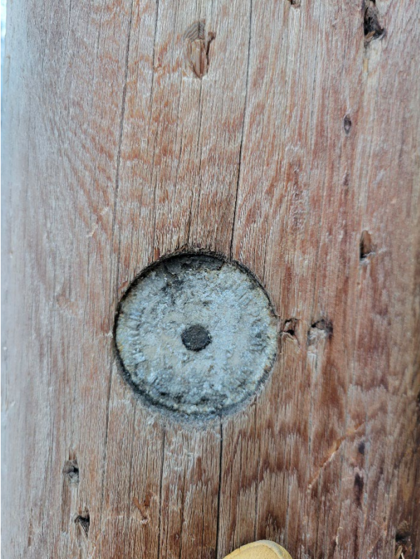
Figure 6. Close-up of faded marker.
