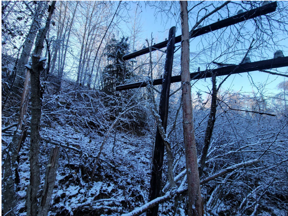
Figure 3. Pole close-up with insulators.
