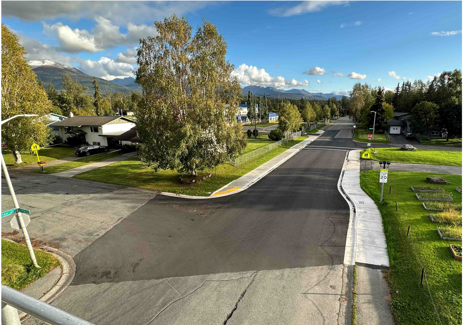
New Sidewalk on Patterson Street and Crosswalk Relocation (Chester Valley Elementary School)
