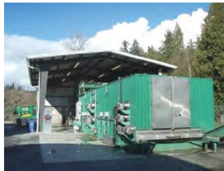
Figure 3-12: Agitated Container System (Wright Digester)
