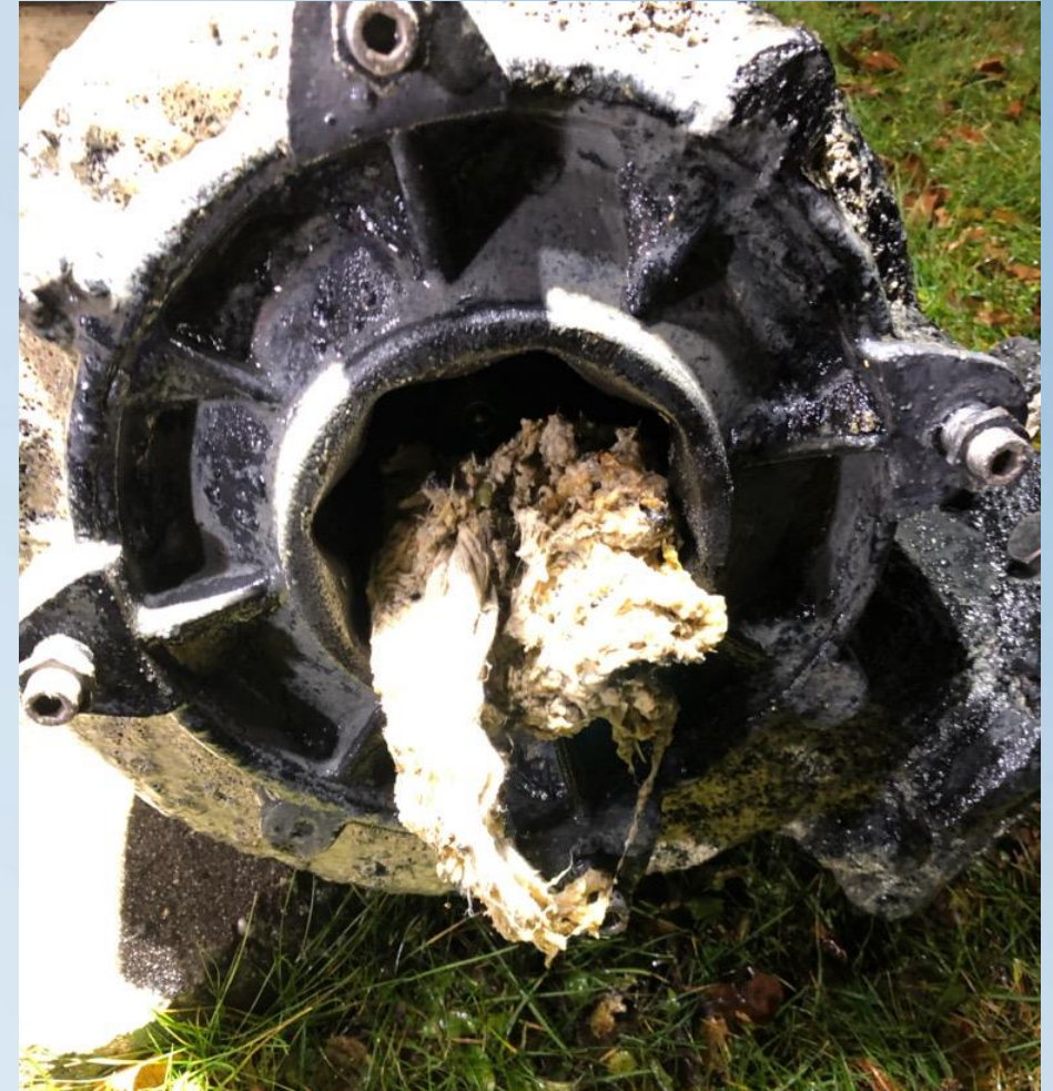
Wipes and diapers plugging an AWWU pump.
