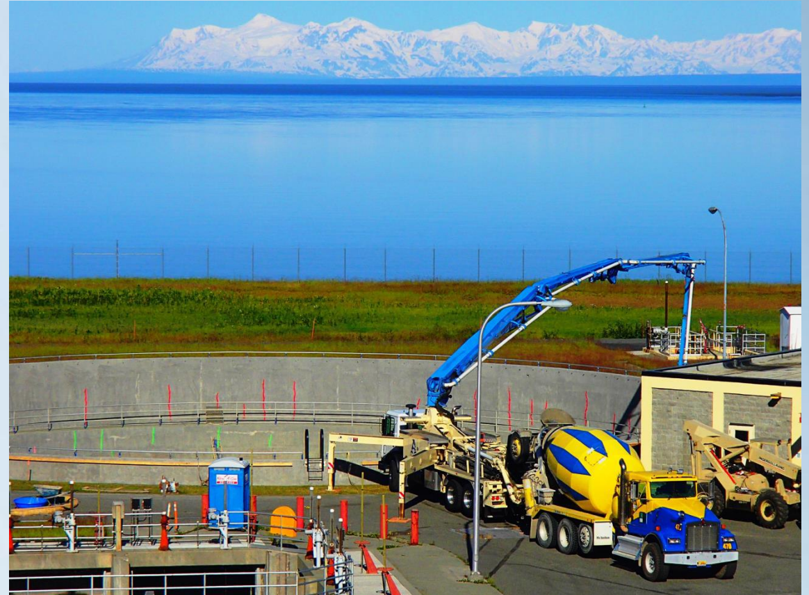
Maintenance on a clarifier tank at Asplund Wastewater Treatment Facility, with the Knik Arm and the Tordrillo Mountains behind.
