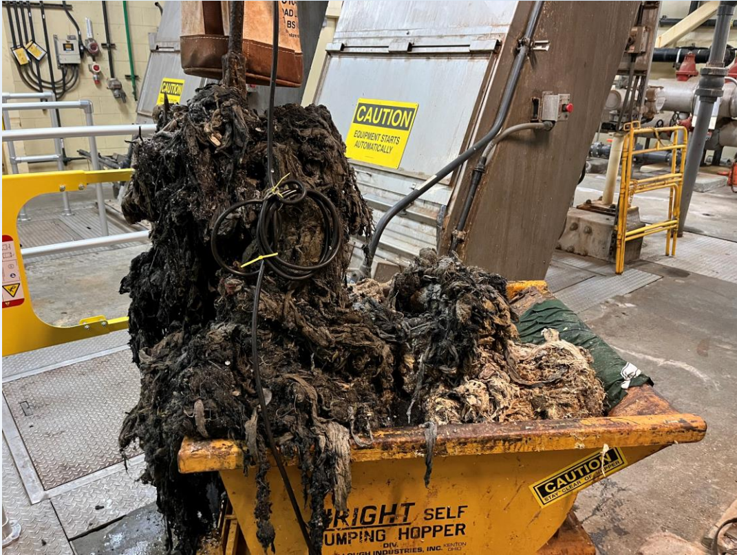
Wipes removed from headworks screens at Asplund Wastewater Treatment Facility.
