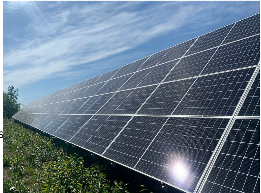
50 kW of solar at the Anchorage Regional Landfill
