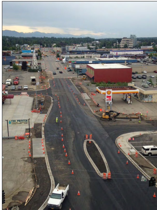
North end of Spenard Road under construction – courtesy of AMATS/Municipality of Anchorage.
