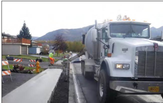
Sidewalk, road, and drainage upgrade on East 17th Avenue. – courtesy of AMATS/Municipality of Anchorage.
