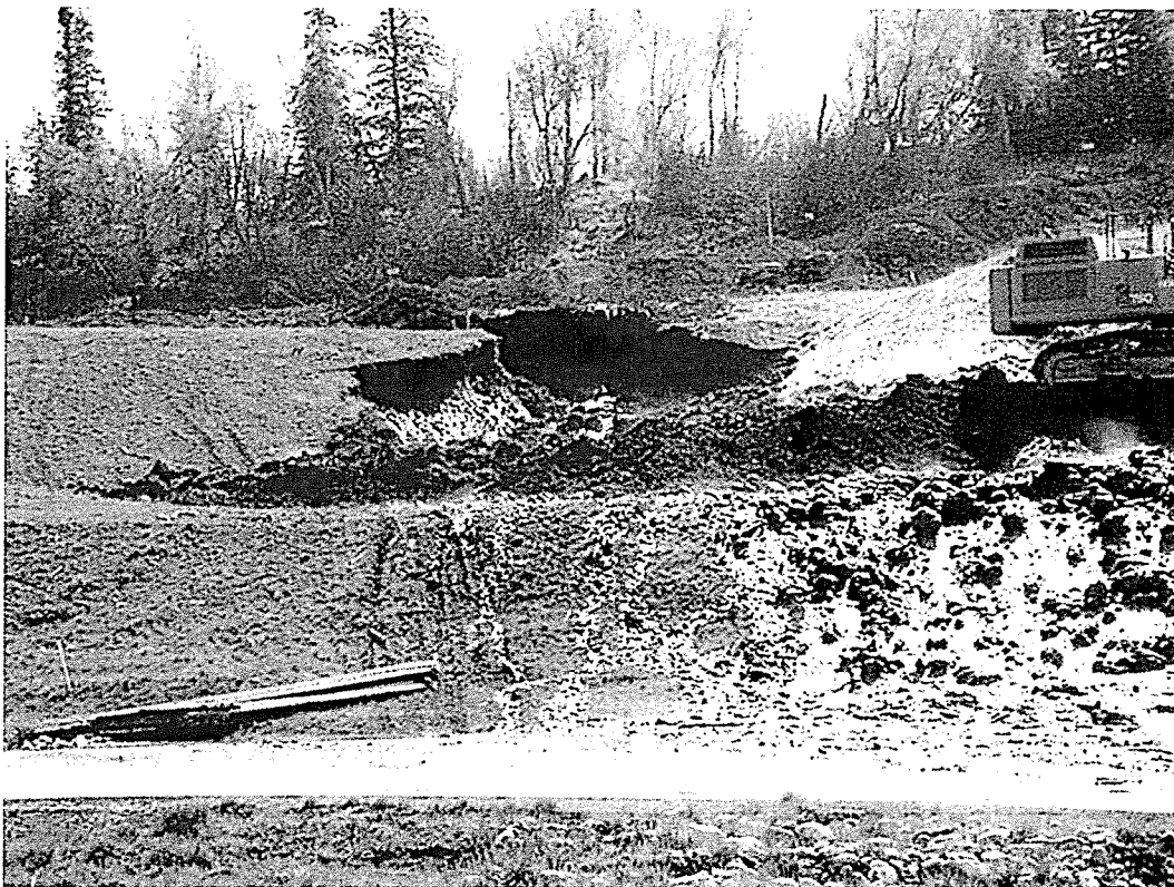
Figure 2. Slope failure near Prominence Pointe on developed slope.
