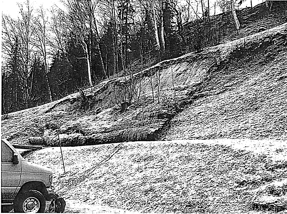
Figure 1. Slope failure on a section of the Rabbit Creek bluff as a result of a property owner clearing and developing steep slopes in violation of Title 21.07.020- (Natural Resource Protection, Section C on steep slope development).
