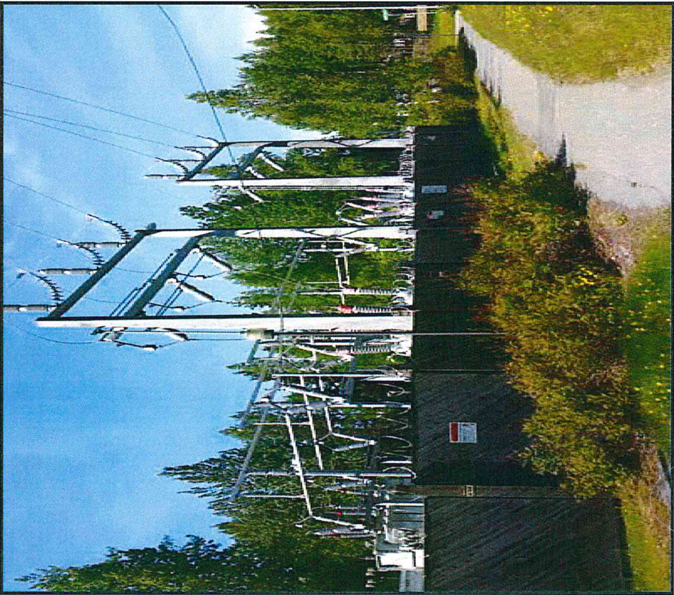
Photo 3 Standing at the Northside of Substation #8, parallel to Northern Lights Boulevard, looking West.
