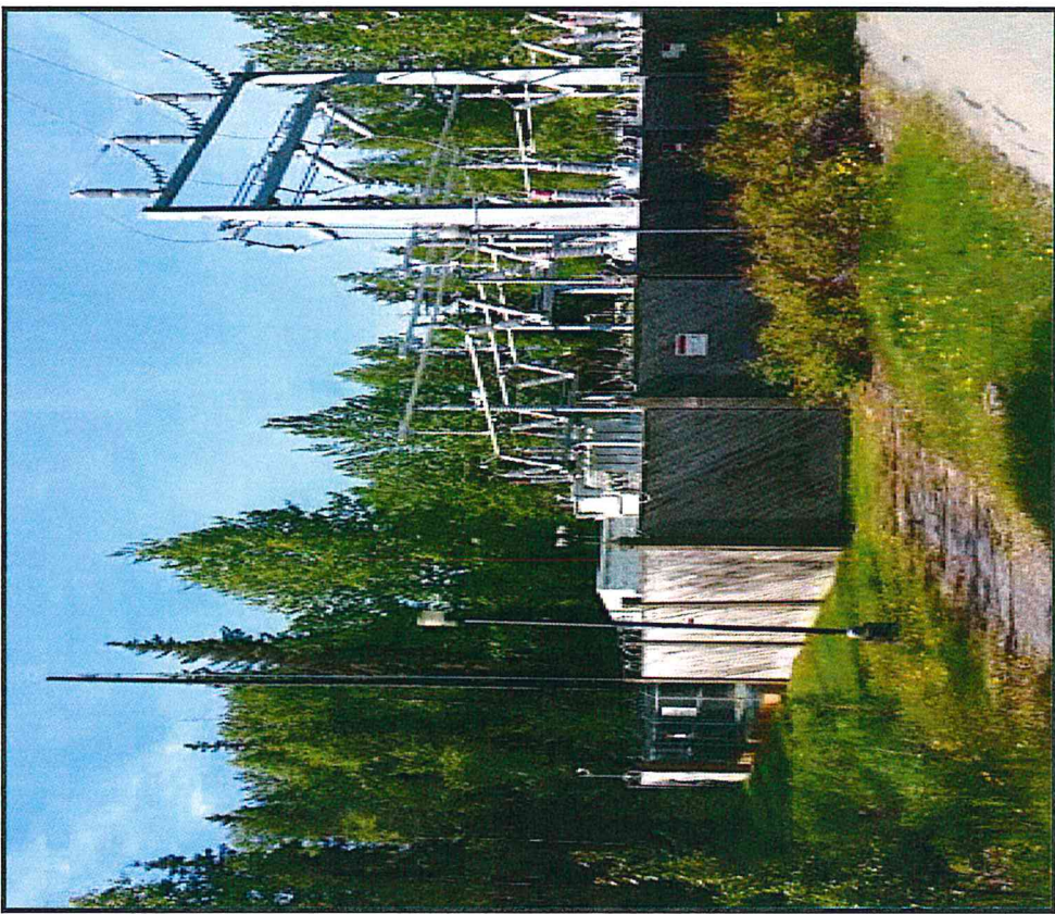
Photo 2 Standing near the Northeast corner of Substation #8, looking Southwest.
