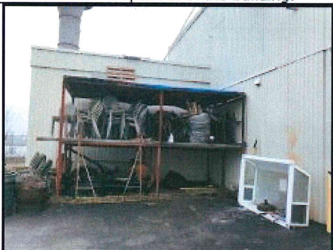
Looking north at the NWC of the building where the addition will be constructed.
