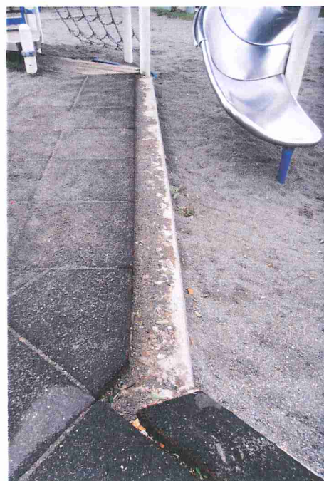
Figure 14 Dated fall surfacing and overflowing pea gravel
