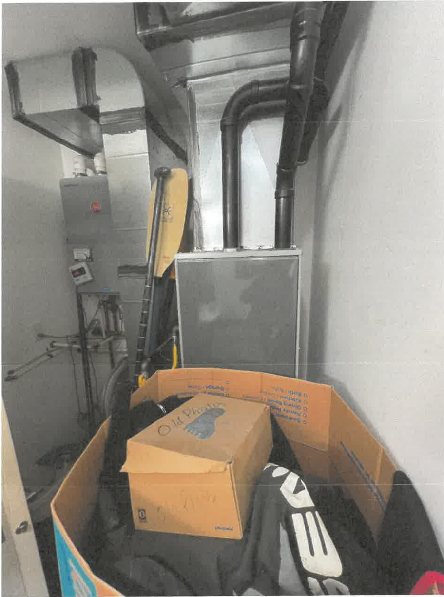
Mechanical room showing furnace, boiler and water shutoff in northeast corner
