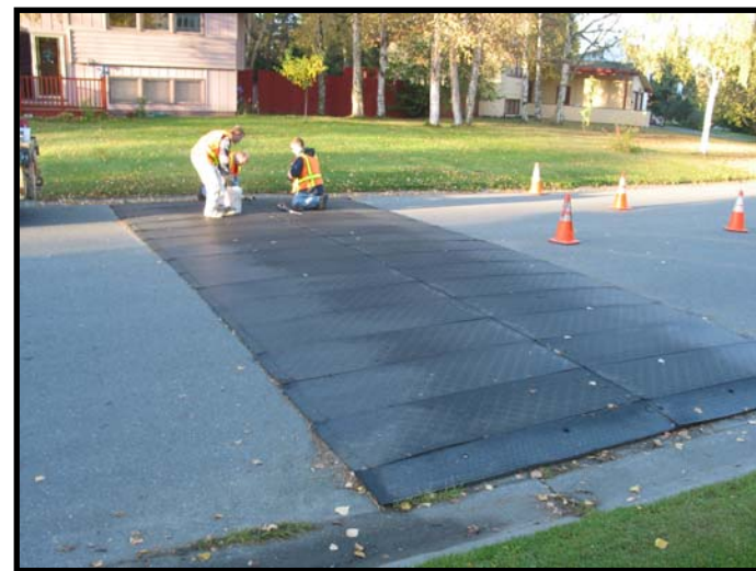
Paint and Sign Shop installation crews work on the placement of a temporary speed hump.
