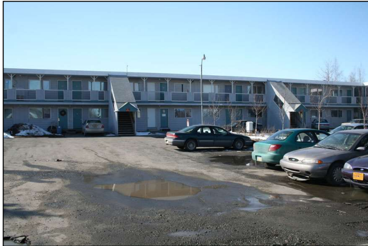
Example of Prohibited External Walkway and External Access Stairway
