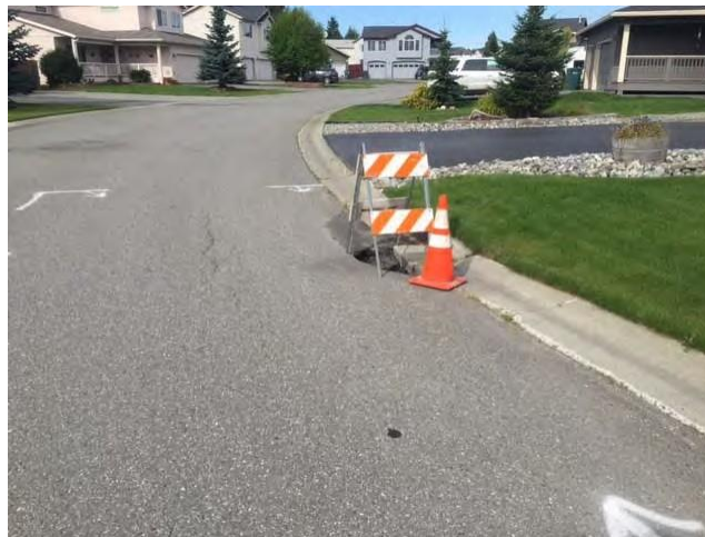
Sinkhole due to failure on Devonshire Circle
