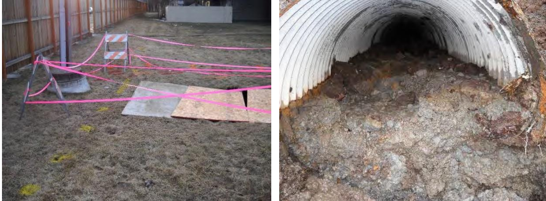
Sinkhole due to pipe failure in a residential back yard off of Canton Loop
