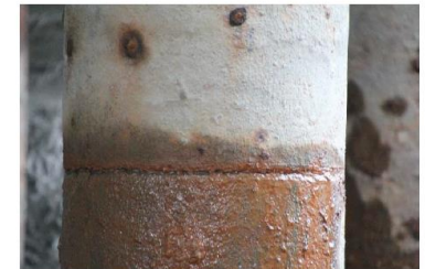
Photo 3 – Pile 3T weeping splice
