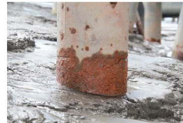
Photo 2 – Pile 1T crack below splice
