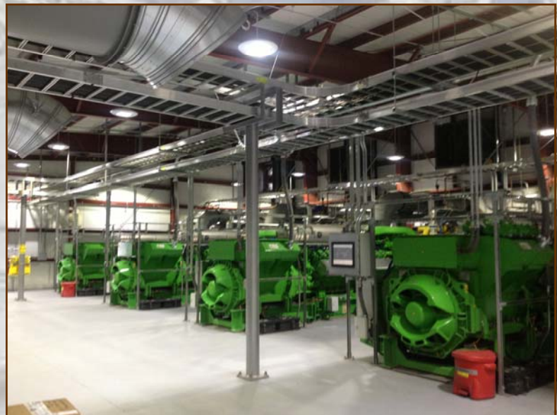
Jenbacher JGS 420 engines at the new Power Plant
