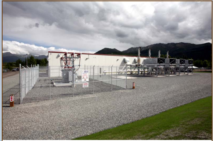
Power Plant transformer and radiant cooling
