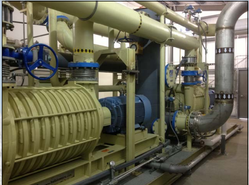
Multi-stage blowers and moisture knock out in GPS Building
